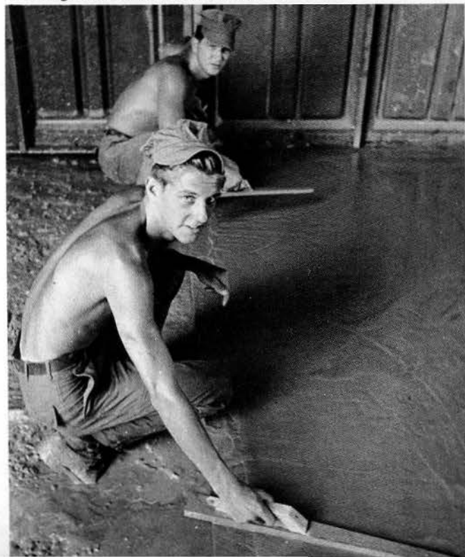
G.J. Furllet, BUR3, (back), and B.E. Furthmyer, BUR3, put finishing touches on a cement floor ▼
