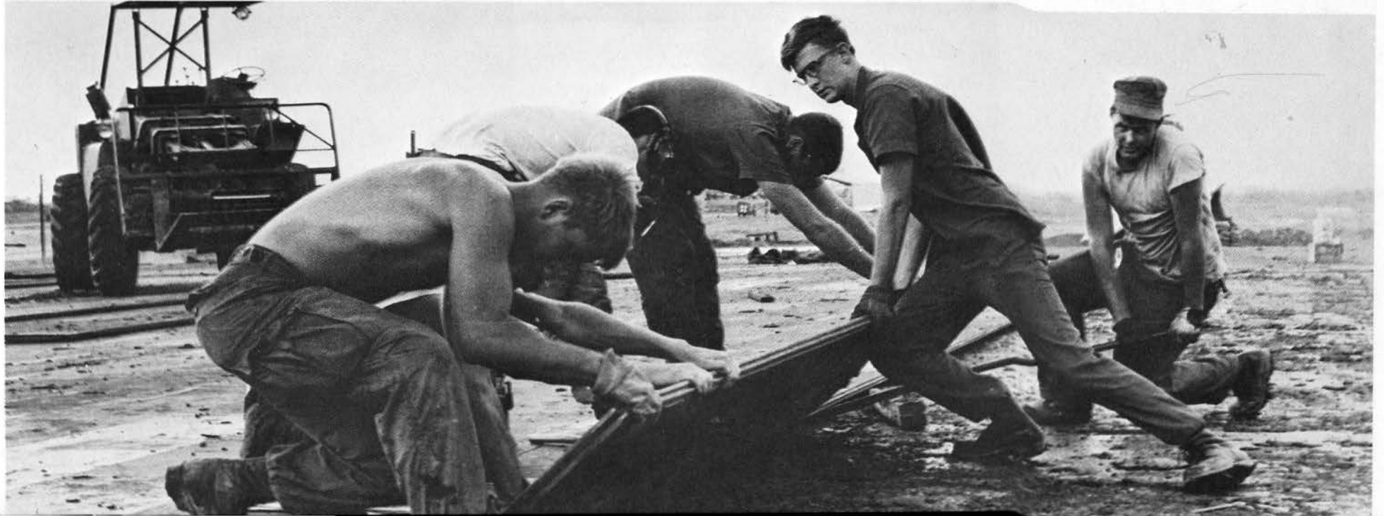
Crew from CBMU 301 "C" Co lays matting at Dong Ha Airstrip to replace section destroyed in rocket attack
