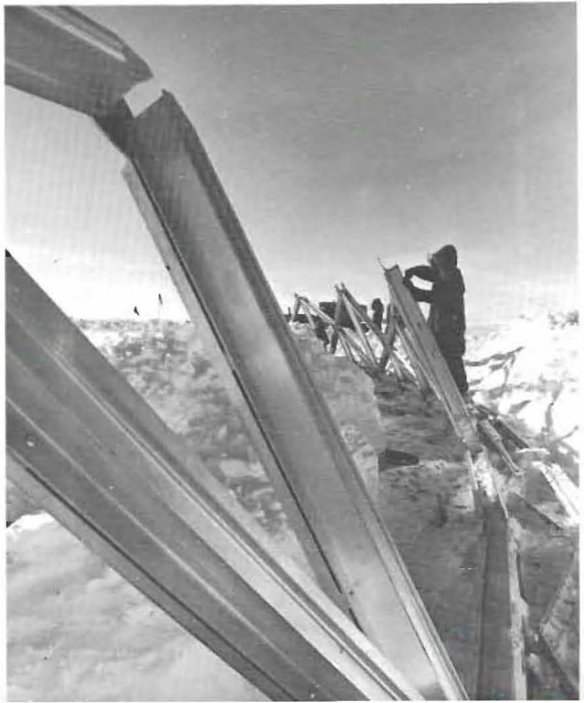
FIGHTING THE ELEMENTS to finish the job on time, a Seabee constructionman works on the framework of the 164-foot diameter dome which will house three of the new station's buildings.
