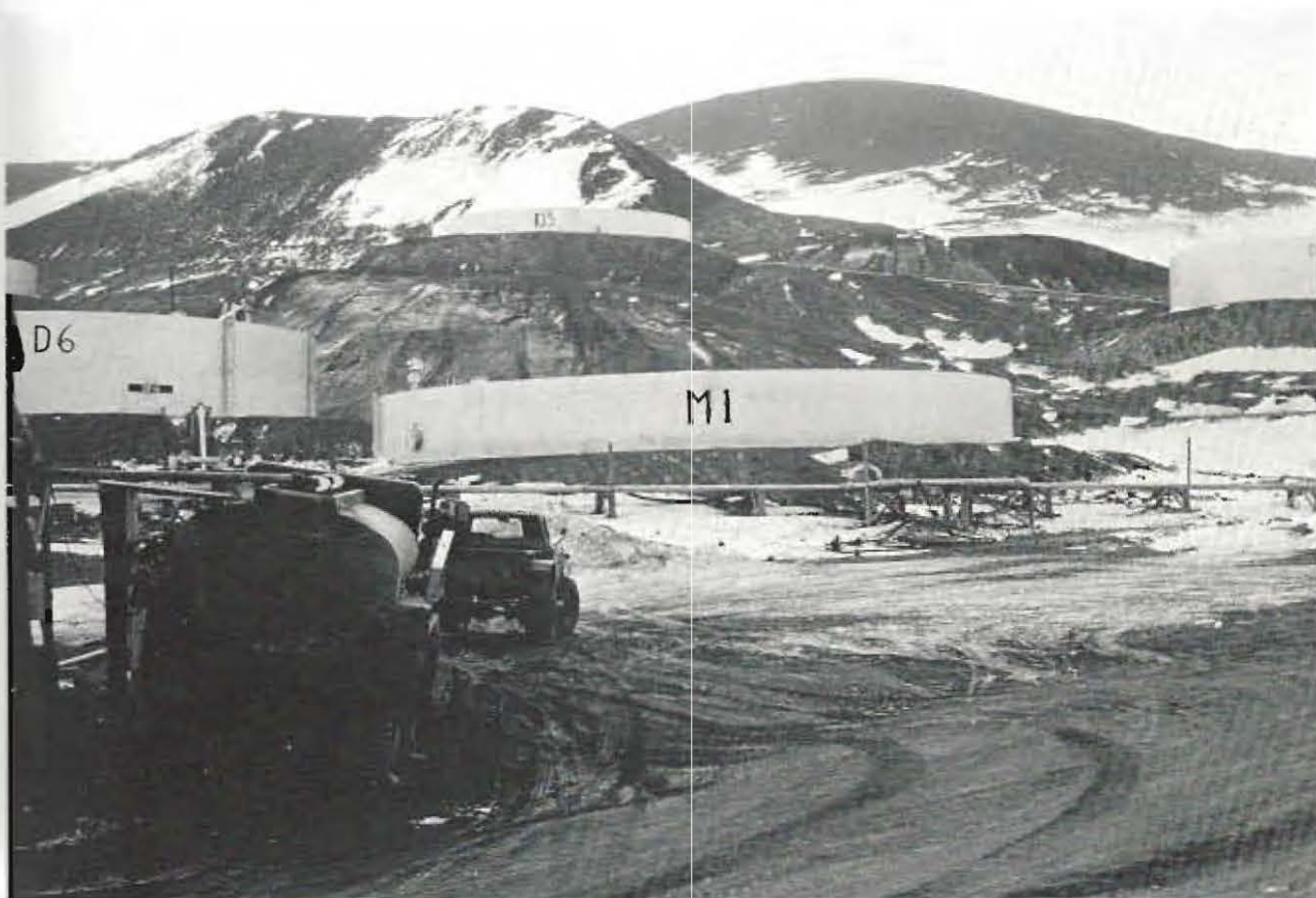
PART OF THE 18-TANK fuel system at McMurdo, the containers hold all the fuel needed to sustain operations at the large U.S. base.
