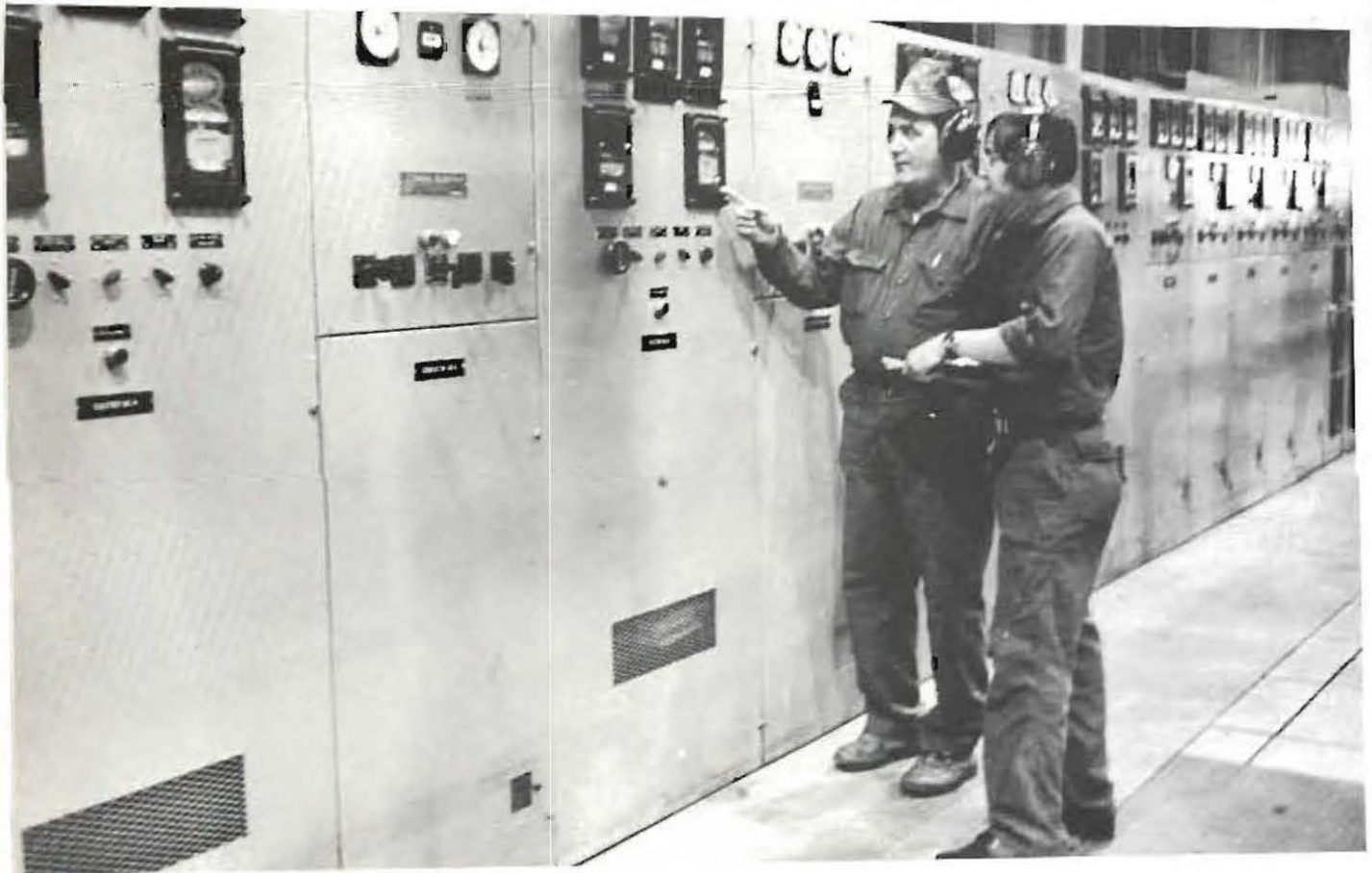
WEARING EAR PROTECTORS to guard against the intense noise level, two power plant operators (BELOW) check the power plant output.
