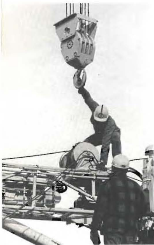
CONNECTING THE RIG to the massive crane (ABOVE) which will raise it upright, a workman attaches the hook to the drill rig frame.
