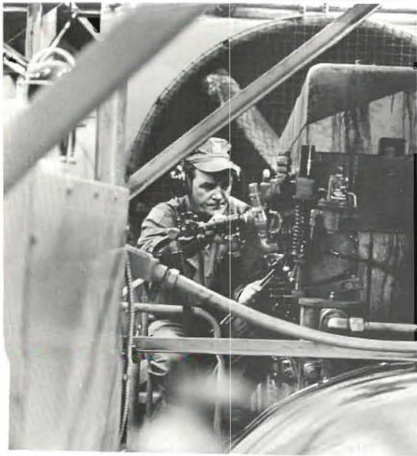
TUNING A DIESEL GENERATOR, Construction Electrician second class Newt Coughenour (LEFT) maintains capability in the power plant.
