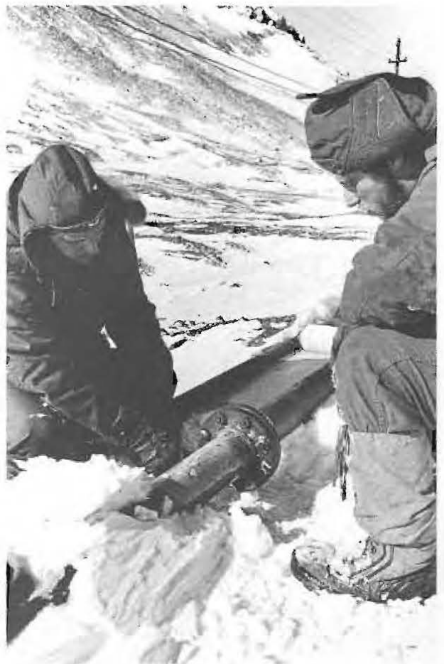
SECURING THE PIPELINE carrying needed fuel to the aircraft at Williams Field, Builders Third Class T. J. Keen (L.) and E. Mroszak apply the proper tension to the lug bolts.
