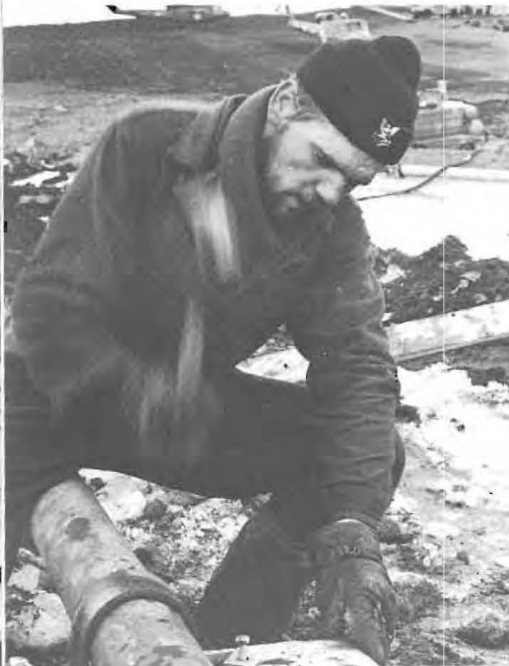
DRIVING A SPIKE to secure a collar holding the helicopter pad fuel line, Builder Third Class Gerard Nault aids in building the line which will improve the fuel supply to the uptown facility.
