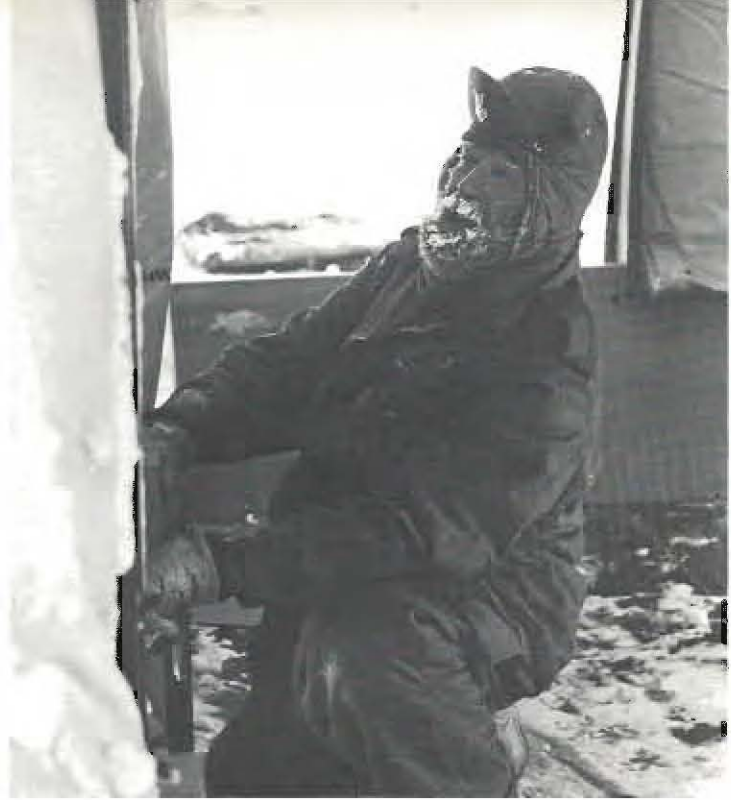
BRACING A DOORFRAME, Builder First Class R. A. Smith (ABOVE) assists in constructing one of the Jamesways at the new station site.
