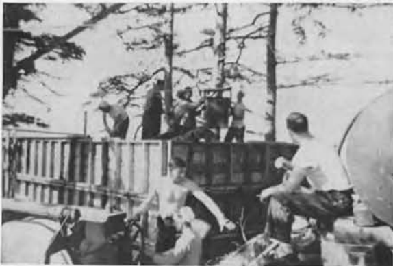
Reading from Top to Bottom: Unloading material. Pouring concrete in shute. Highline between islands. Concrete shute. Concrete crew at work.
