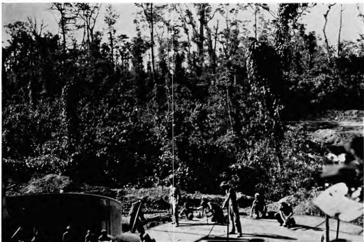
We moved tanks out of jungles and built others in more jungles.
