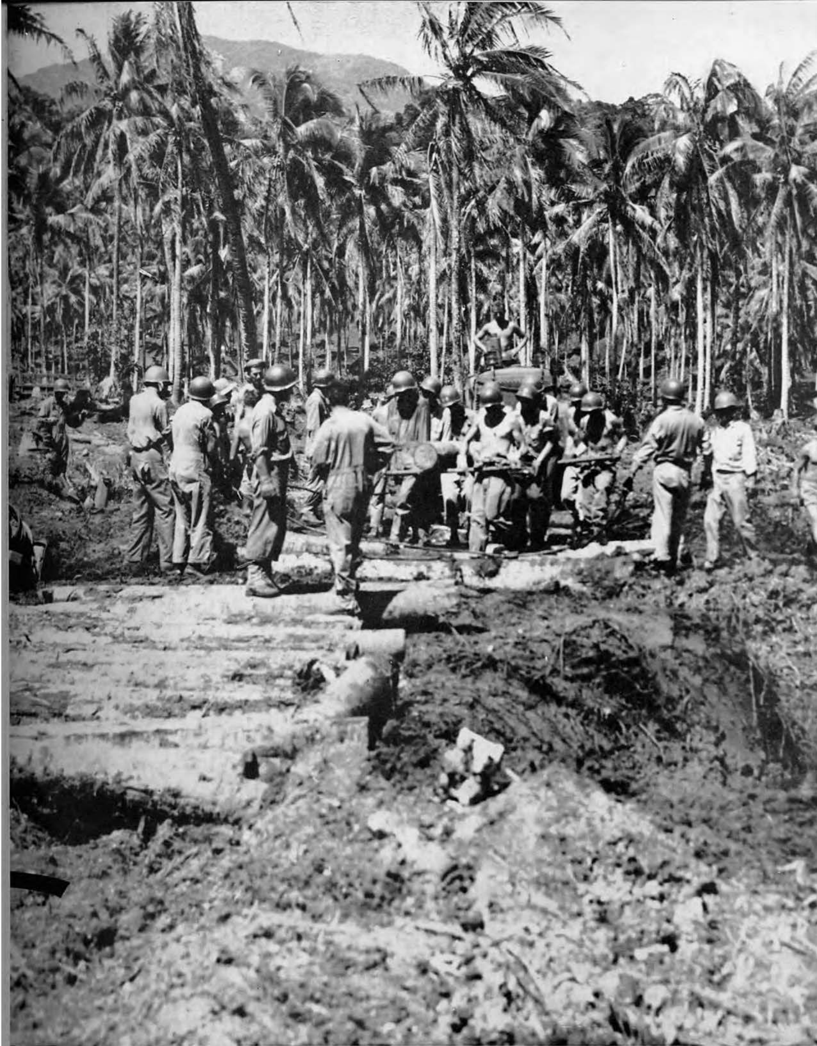
A log road is made through the jungle mud on Rendova Island. Coconut palms felled along the route served as a ready supply of road building material. Heavy artillery of the Marines was carried over this road to a point where it was in range of the Jap stronghold at Munda.
