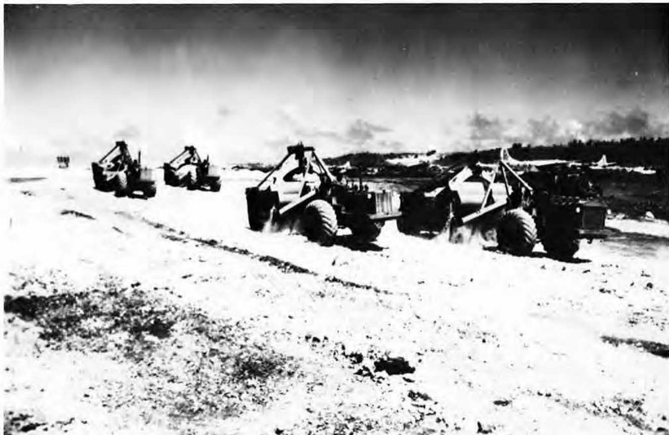
Heavy scrapers cut down hills and moved the coral to fill in depressions at North Field. Surveyors checked proper grade throughout the work. Photo, Norman Symons.
