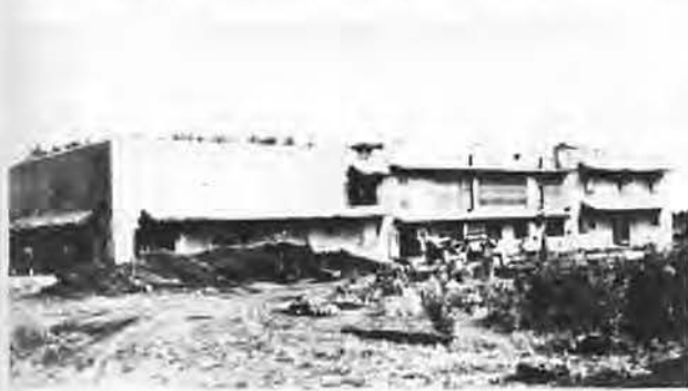
Damaged Japanese Command and Communications Center. The concrete structure survived concentrated gunfire. Photo, Norman Symons.
