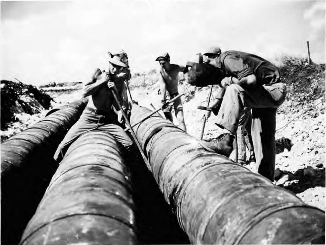
Seabees welded together empty 55-gallon fuel drums to build a drainage system at North Field. Pipes ran under the runways and taxiways to prevent collected water from endangering operations. Photo, Frank Schmidt.
