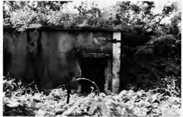
Japanese bunker with shell damage. Photo George A. Larson.
