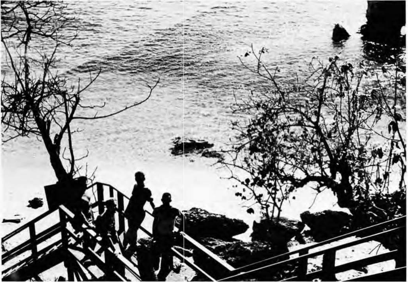
Seabees built stairs down to their beach area on Tinian. Photo, John Vandervort..
