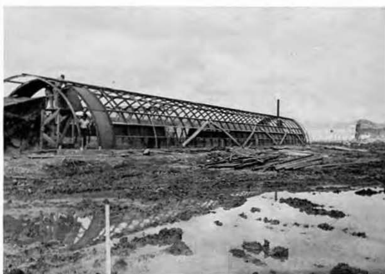
Construction of facilities at the Yonabaru airfield was one of the 145th's biggest jobs on Okinawa. This project included the erection of eighteen 20 by 56 quonsets and three 40 by 100 quonsets; construction of one hundred 14 by 14 tents with framing and wall, and construction of one hundred 16 by 16 tents in the same fashion; construction of a 40 by 200 foot wood terminal building; a one thousand man mess hall and galley; and installation of electric and sewage systems. Upper photo shows the tent area; lower photos, the quonsets under construction. These facilities were completely wrecked in a typhoon that hit the island on October 9th, and had to be rebuilt.
