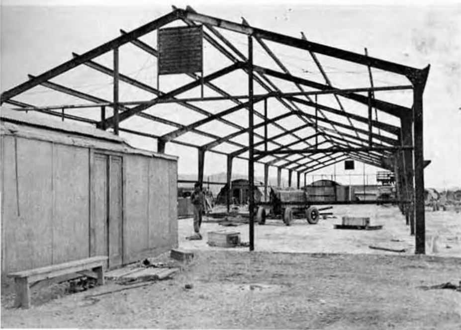
Pictured here is a new type of steel frame construction the 145th used to replace the terminal building at Yonabaru.
