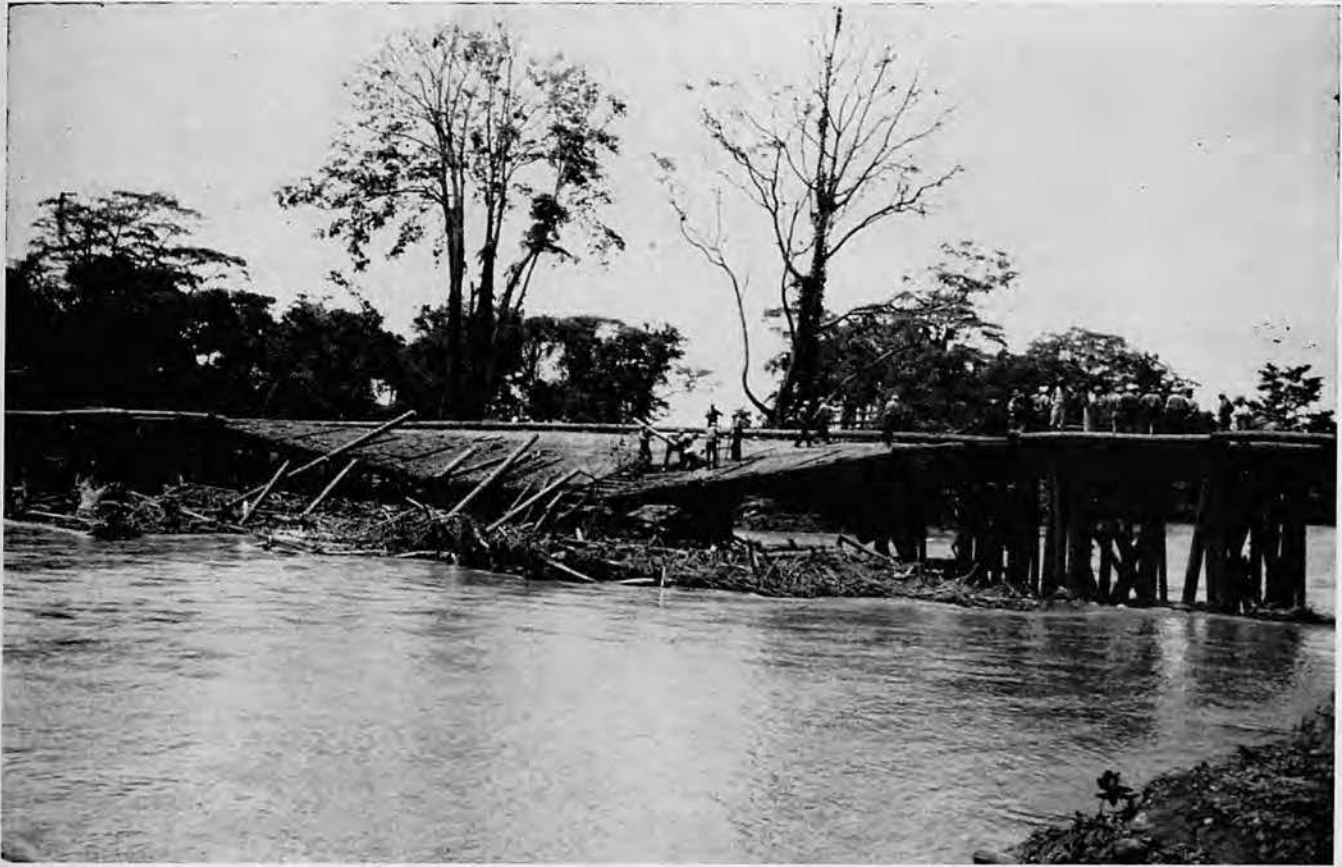
The original timber bridge after the flood had subsided.
