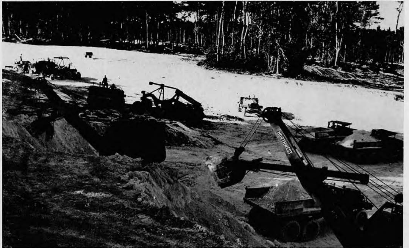
Shown above: Heavy equipment busy hauling coral for a highway fill. Lower: Shovels dig coral for taxiway construction.
