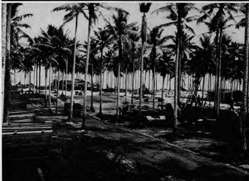
In the upper picture, 27th Battalion men are shown stacking pipe. The lower picture covers a section of the lumber yard.
