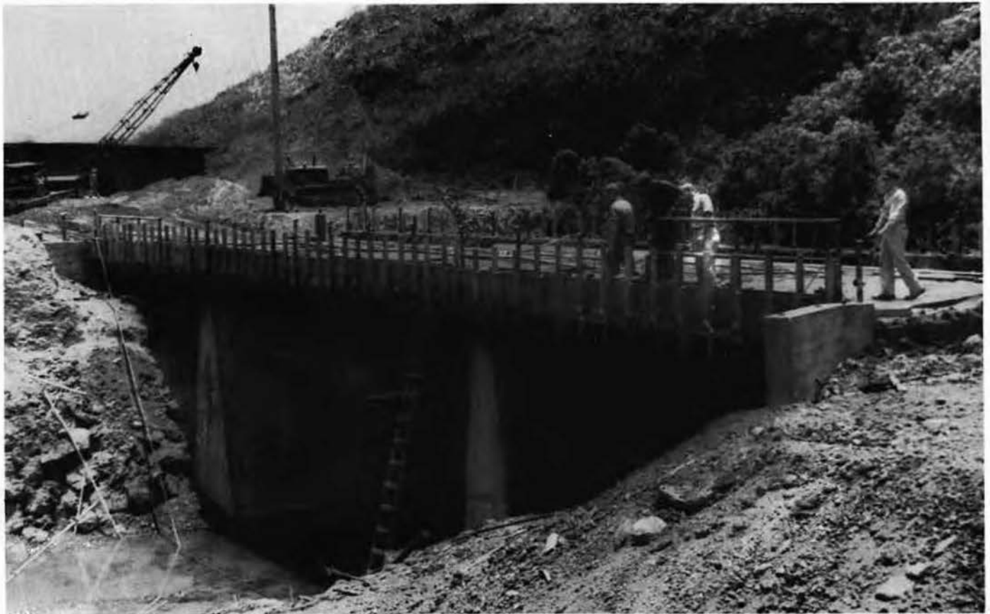
REINFORCED STEEL AND CONCRETE COMPLETES THE BRIDGE FOR HEAVY NAVAL SUPPLY LOADS
