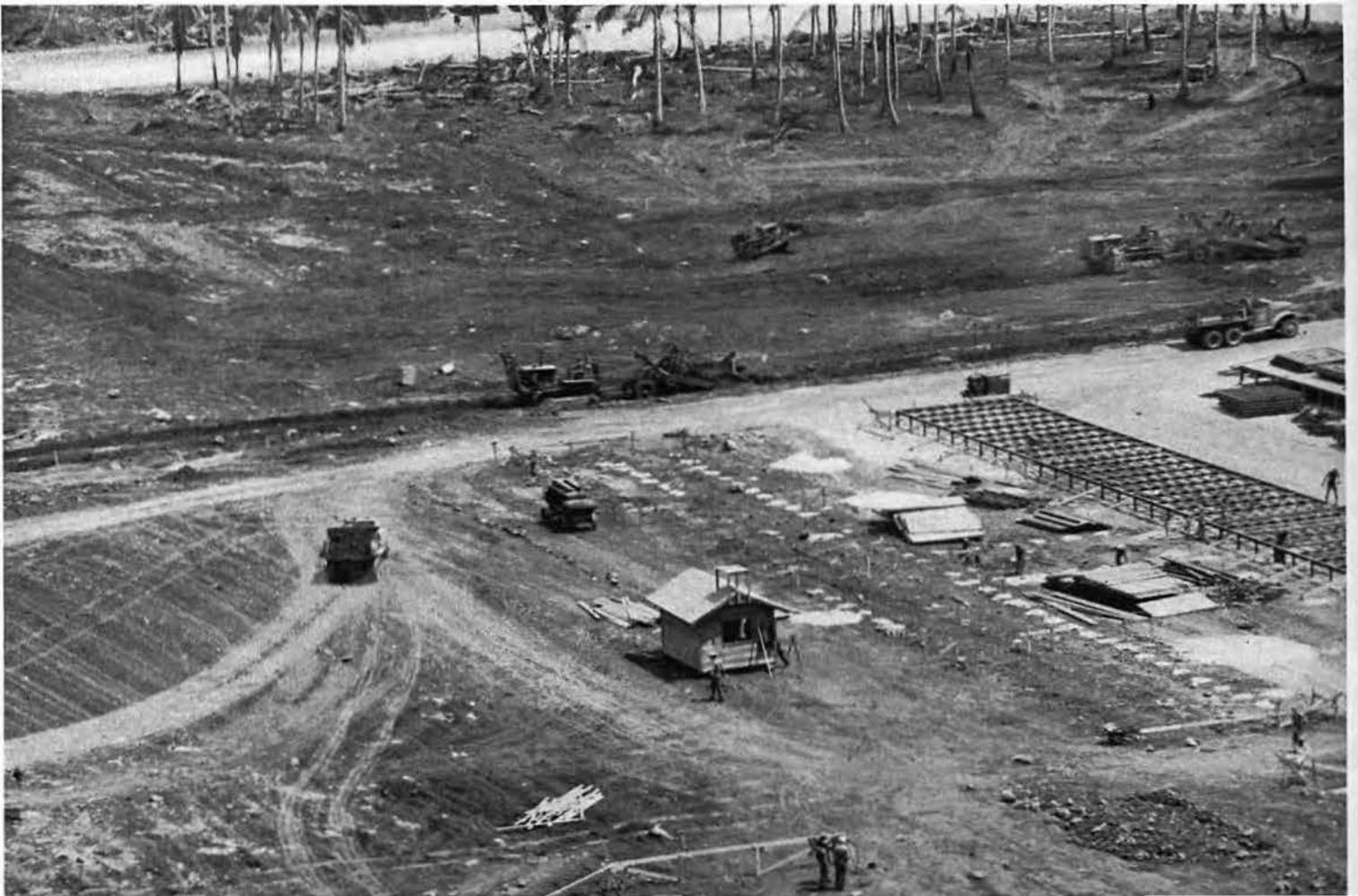
Excessive heat and intermittent Philippine rains hampered construction in all its phases, but credited supervision and high enlisted morale built against a dead-line.
