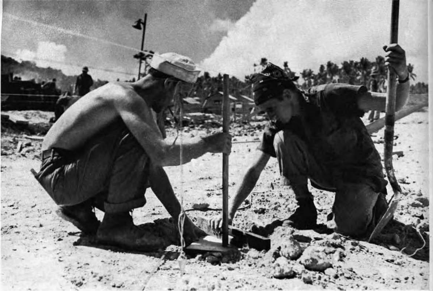
Many men worked in the boiling sun; over dazzling coral, laying footings for 36 Task Force type Ward Buildings.
