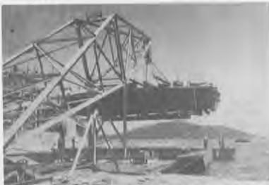
The 75-ton crane can lift a P.T. boat out of the water.
