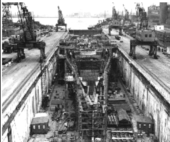
Battleship Kentucky (BB-66), the sixth and last of the Iowa class battleships, sits incomplete at Norfolk Navy Yard-Portsmouth, 1946. The Navy eventually launched her incomplete and scrapped her a few years later. The boilers for the ship were placed in the fast replenishment ships USS Camden (AOE-2) and USS Sacramento (AOE-1) and a section of the bow was placed on USS Wisconsin (BB-64). (U.S. Navy photo)
