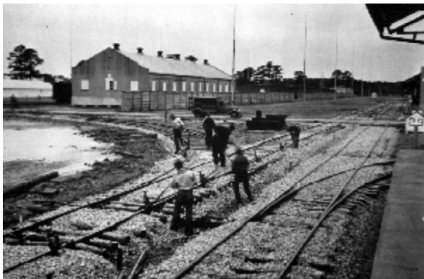
A maintenance of way gang works on of the main railroad lines at St. Juliens. The Hampton Roads facility had an extensive railroad network that connected to the area's major railroad lines to move supplies and completed ammunition. (U.S. Navy photo)
