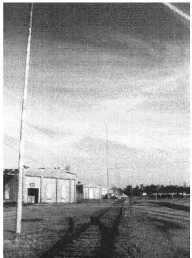
A picture of St. Juliens Creek Annex’s lightning rod system. Boring? To some, yes, but to others it is fascinating. More importantly, the interest value is not nearly as important as its interpretive value.
