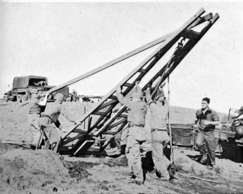
The canteen full of water which the men brought with them will not last very long. So, Chief SELLERS and his utility shop crew, erect a derrick and drive a pipe down to water level.
