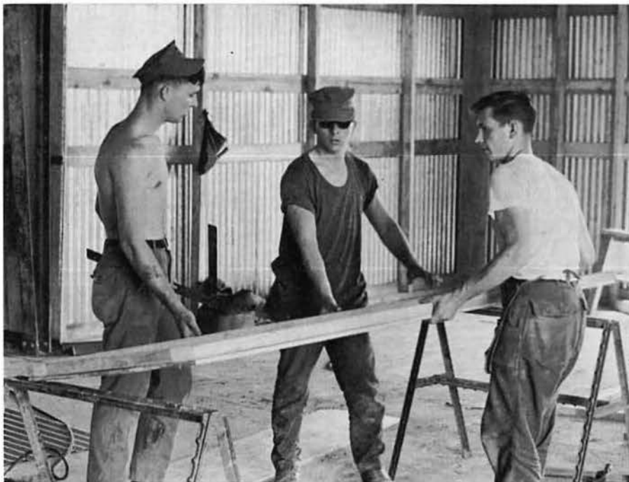
BUR2 WHITTLE, BULCN KERN and BULCN LLOYD laminate a door in the new Bravo and Charlie Company Shops.
