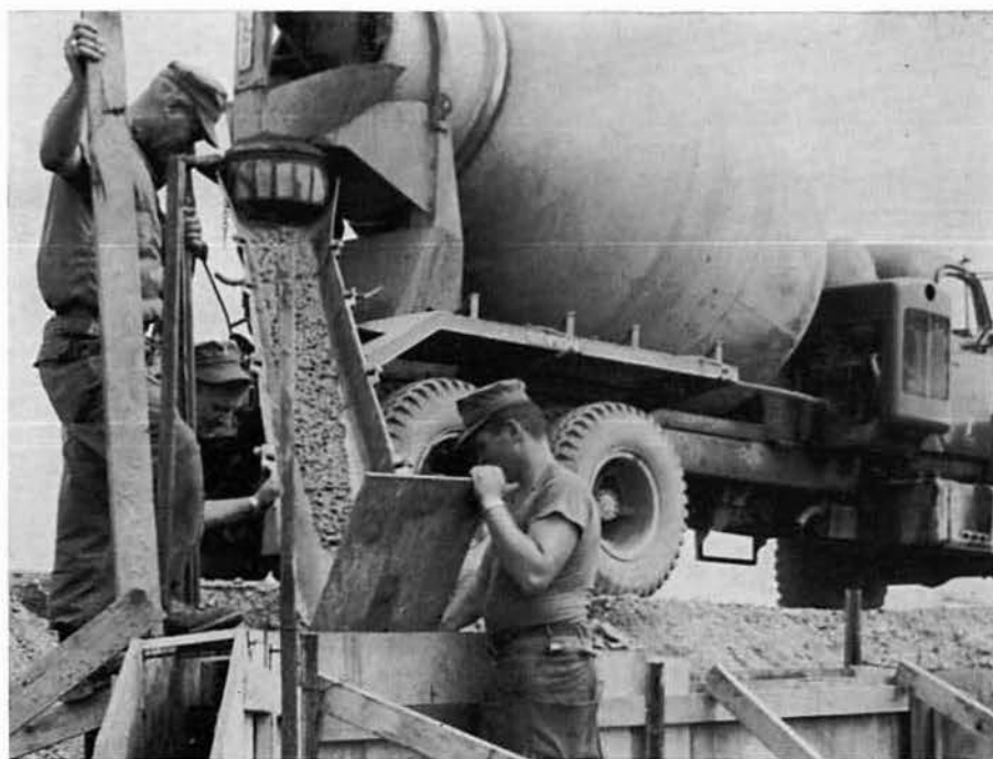
BUL2 WEBBER, BUR2 WHITTLE and BUR2 THRONSON construct a culvert opening near the Dong-Ha Airstrip.
