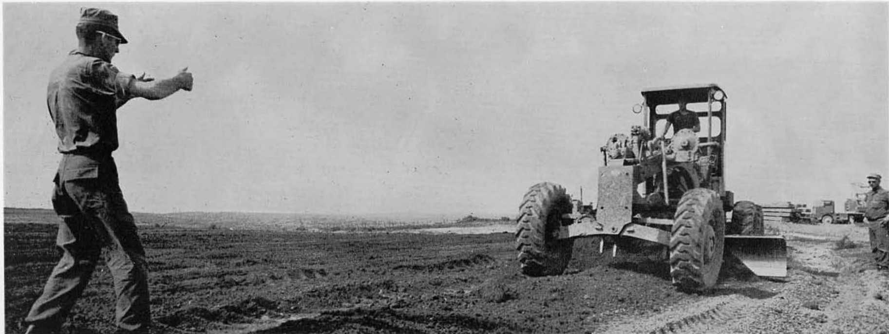
EO1 HED guides the road scraper operated by EON3 WOODS . EOC BERTLES supervises the grading for the CTR grounds.
