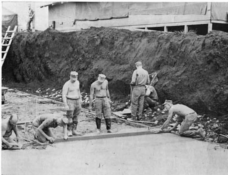
BUL2 SHUGART, EON2 SILER, SWC NUNNELLY, CMA2 CLAIR and BUH2 SEVERIN lay a concrete slab for an underground bunker.
