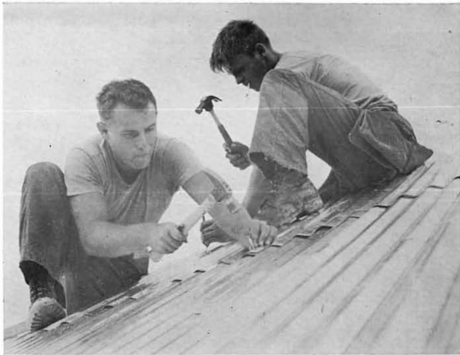
BUR3 STRUIK and BUH3 SUNDSTROM construct a tin roof for a camp hooch.
