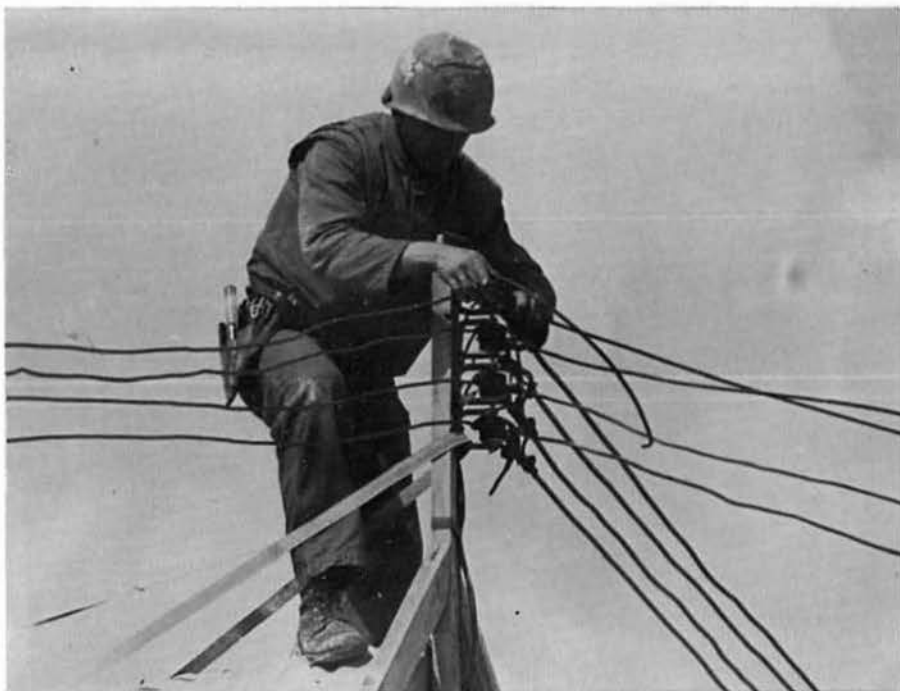
CEP3 QUIRING repairs power lines at Delta Med after shrapnel severed the cables.
