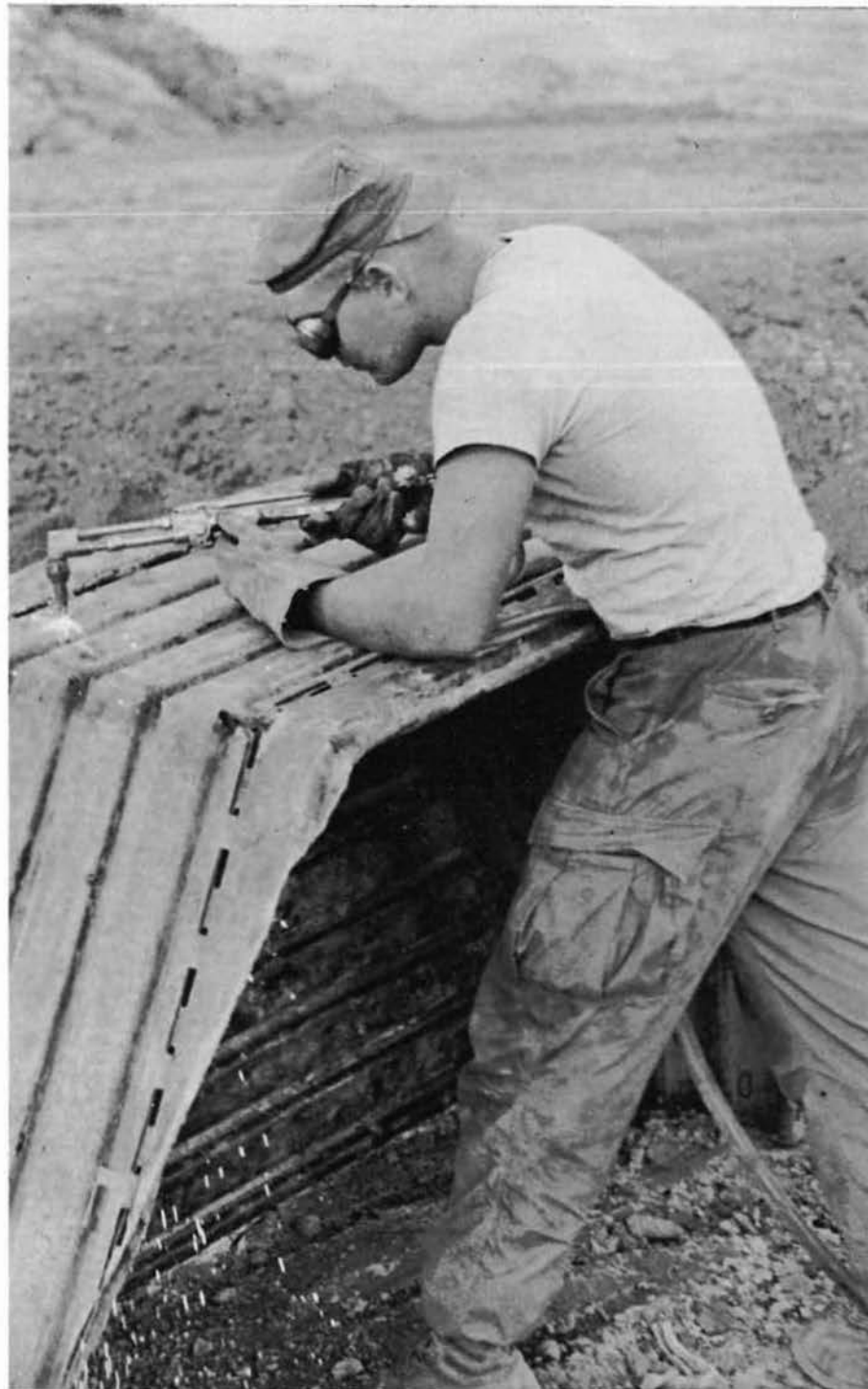
SWE3 BORTMAS welds a headwall made of runway matting for one of the camp culverts.
