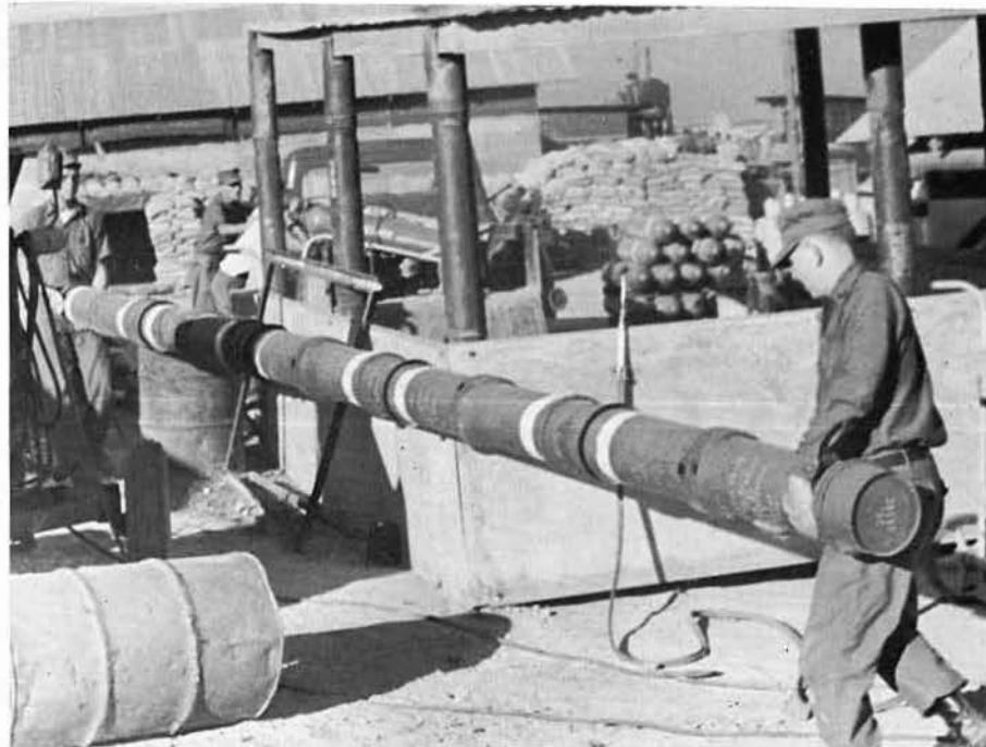
CEP2 DIBELKA and CET2 ULMER carry a cannister power pole out of the steelworkers shop.
