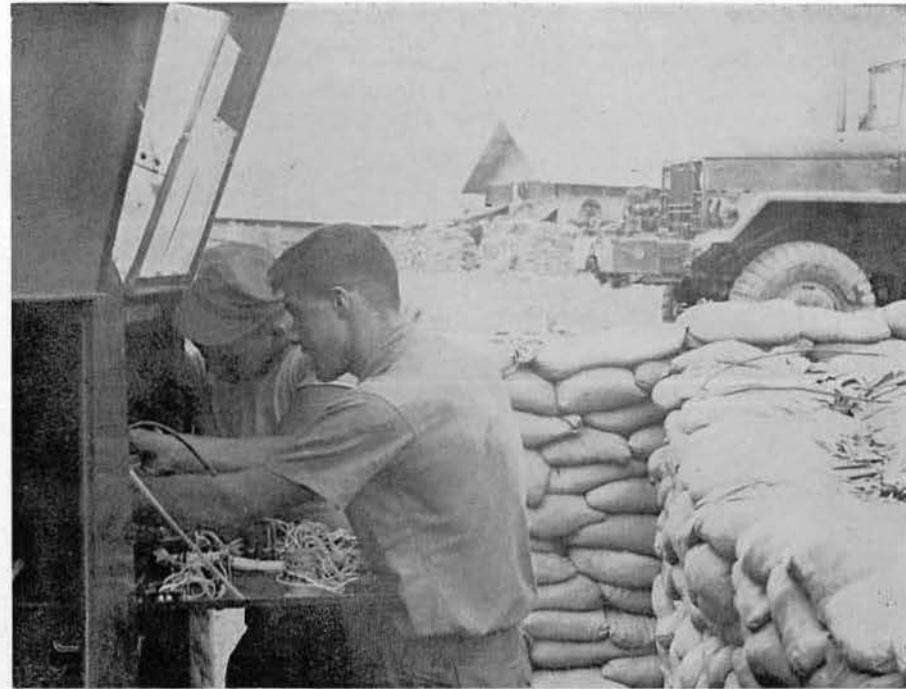
CMHCN COCHRAN and EON3 GLYNN work rapidly to get the camp's power generators back in operation.
