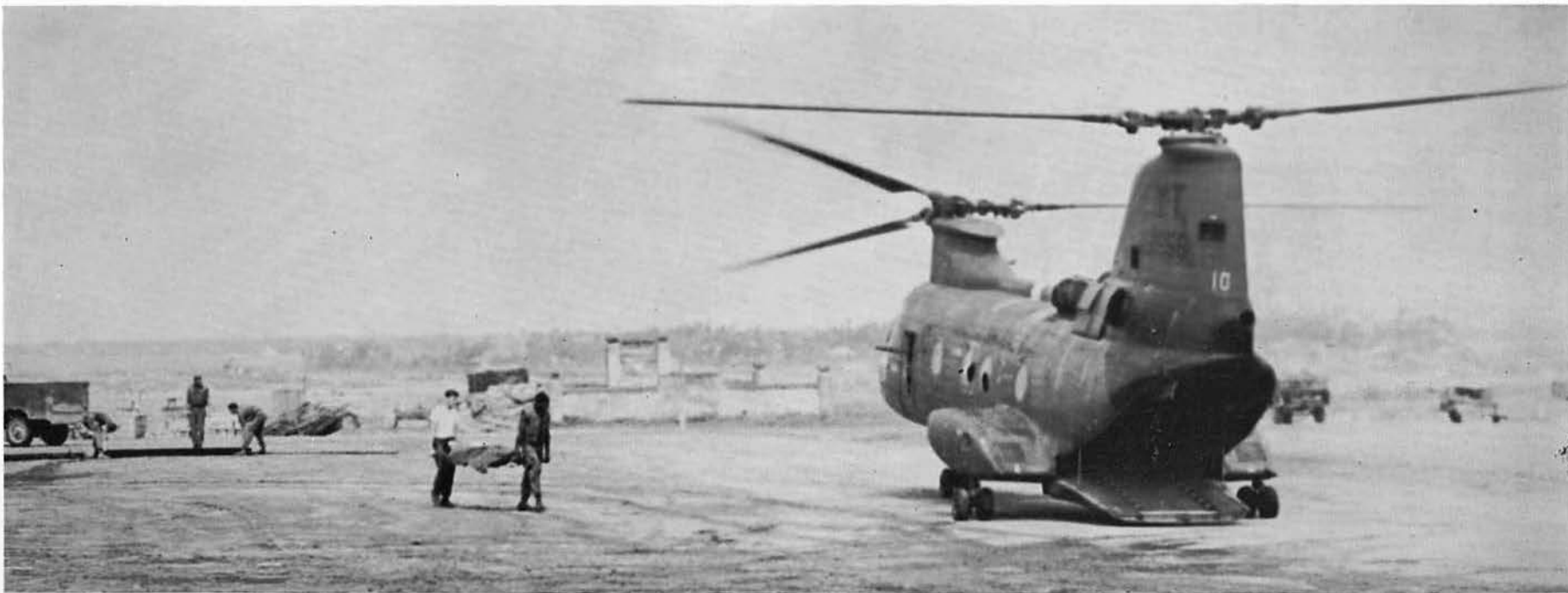
Steelworkers lay matting on the Delta Med helipad as a Seaknight stands by for a medevac.
