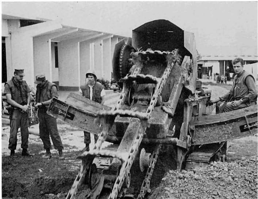
Lt. (jg) MONTI, Ens. ROEN, EONCN ALEXANDER and EON3 THIEVERAGE. The trencher is constructing ...
