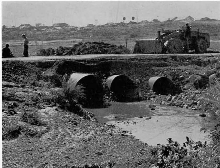
CBMU 301 seabees work on a road culvert at the end of the Dong-Ha Airstrip.
