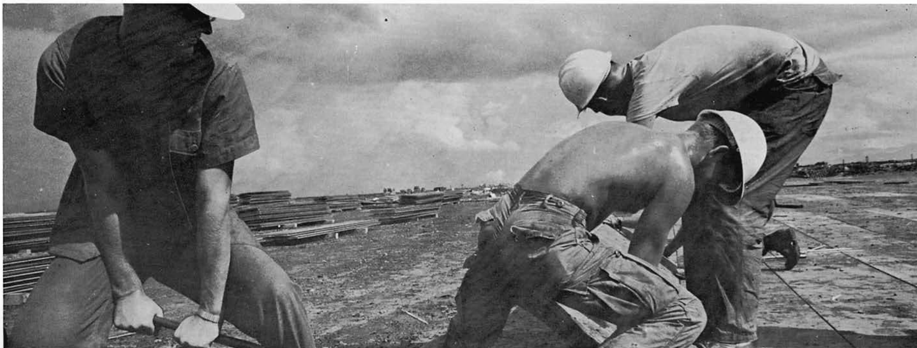
CN WILSON, SWE3 CROW and SWE3 SEDILLO place matting on the Dong-Ha runway. This was one of the steelworkers main responsibilities.
