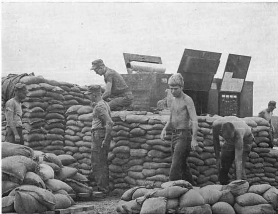
Sandbagging the camp generators. CN SHEARIN (center) looks for a square bag.
