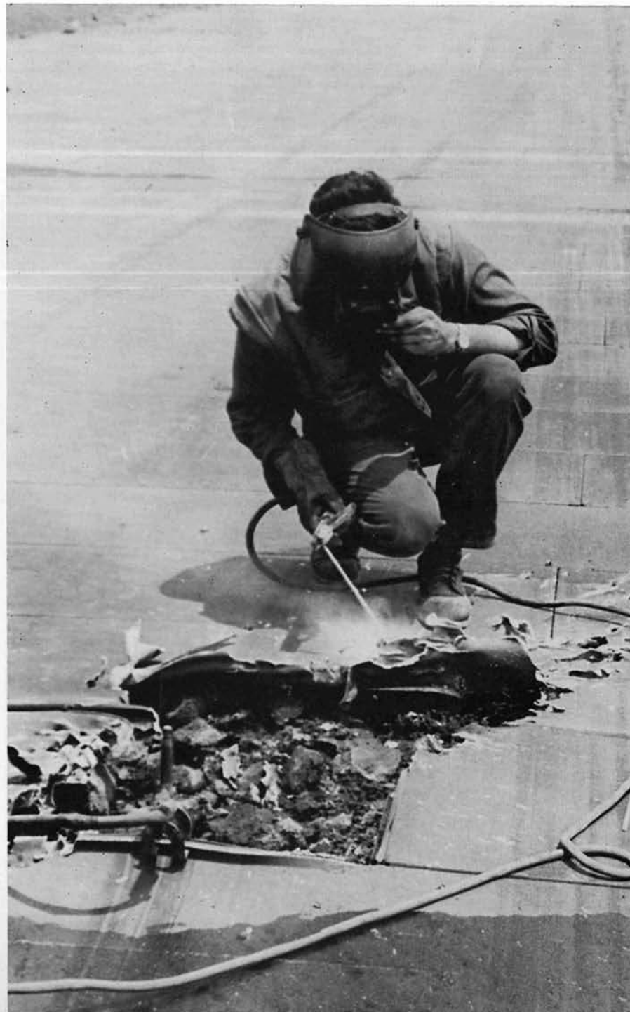
A steelworker cuts the sections of matting damaged by an enemy artillery round.
