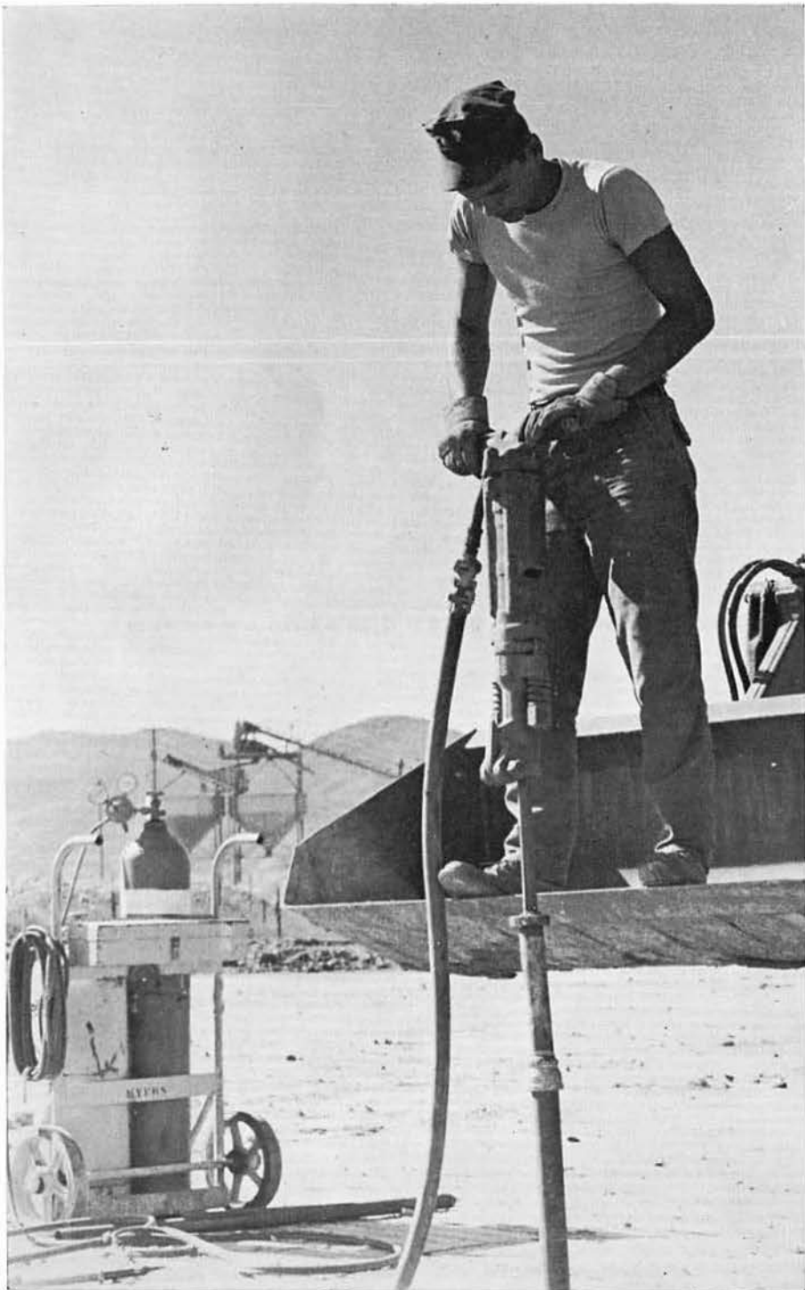
SWE2 PRATT stands on a front end loader to drill an anchor hole in the matting.
