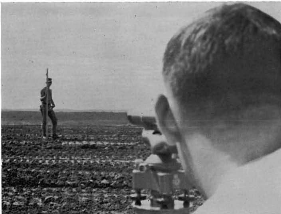
EAS3 BOLTON steadies the rod as EAS2 JOHNSON sets a level for the CTR butler building foundation.
