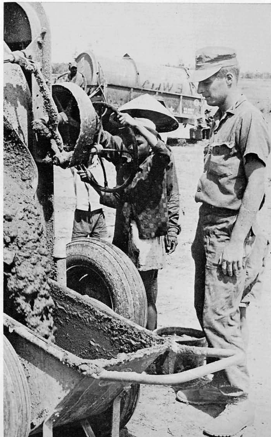
The villagers of Dai An operate the concrete mixer under the supervision of BUR2 CAPPs .
