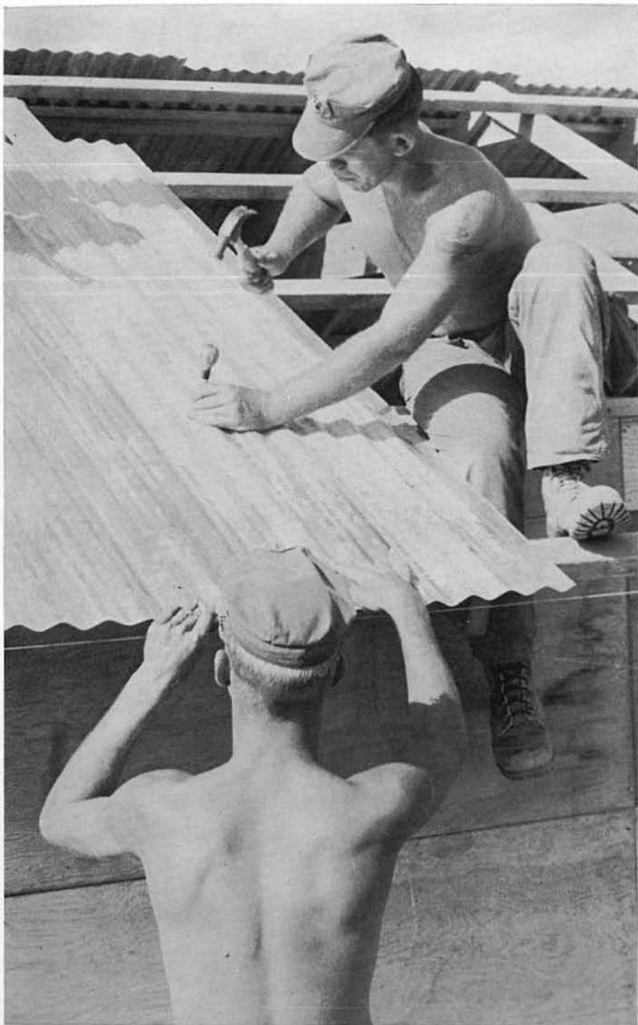
BUL2 HANEY and BULCN McCOMBS tin the roof of the Charley Co. Shop.
