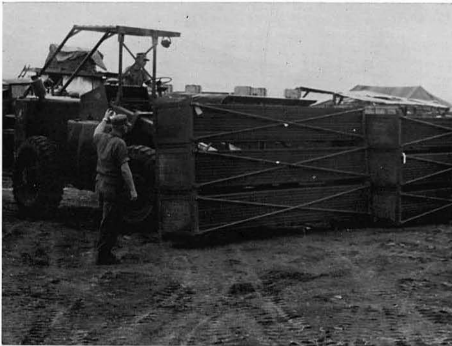
Guided by EOC REES, EON3 BROKAW places a stack of AM-2 airfield matting.
