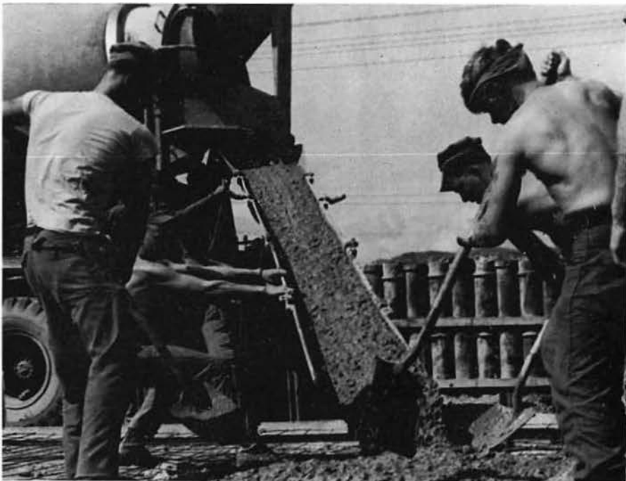
BUH3 SUNDSTROM, BUL3 MATTHEWS and BUL2 LUEBBEHUSEN pour the floor of the new sick bay.
