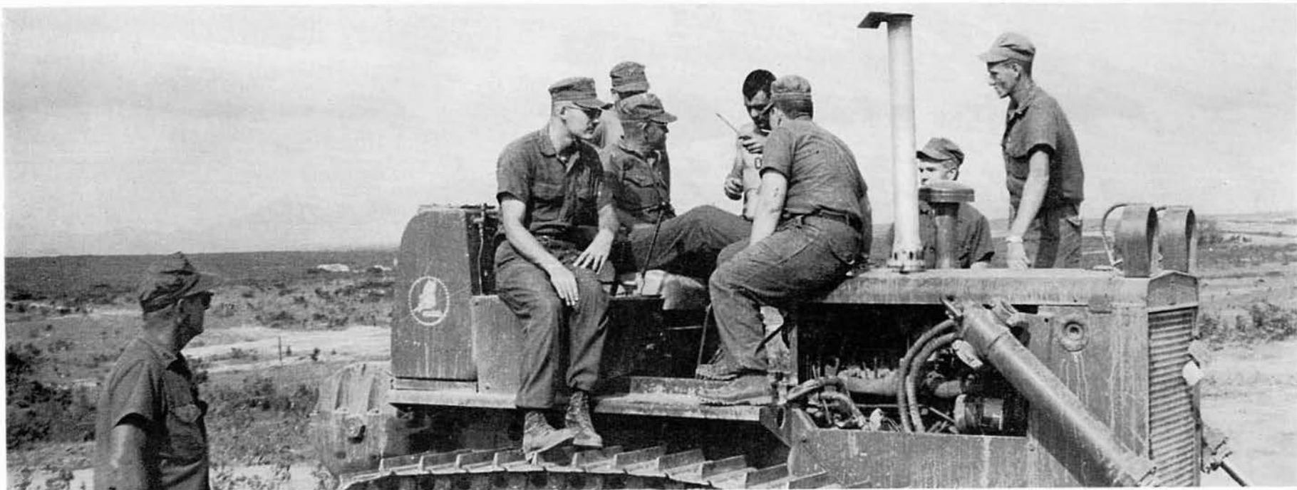
BUL2 SHUGART, Lt. (ig) MONTI, EON2 MORTON, BUL3 KELLY, EAD3 REISTAD, and BUH2 JONES supervise the work of CM1 DOUGLAS attempting to repair a dozer.
