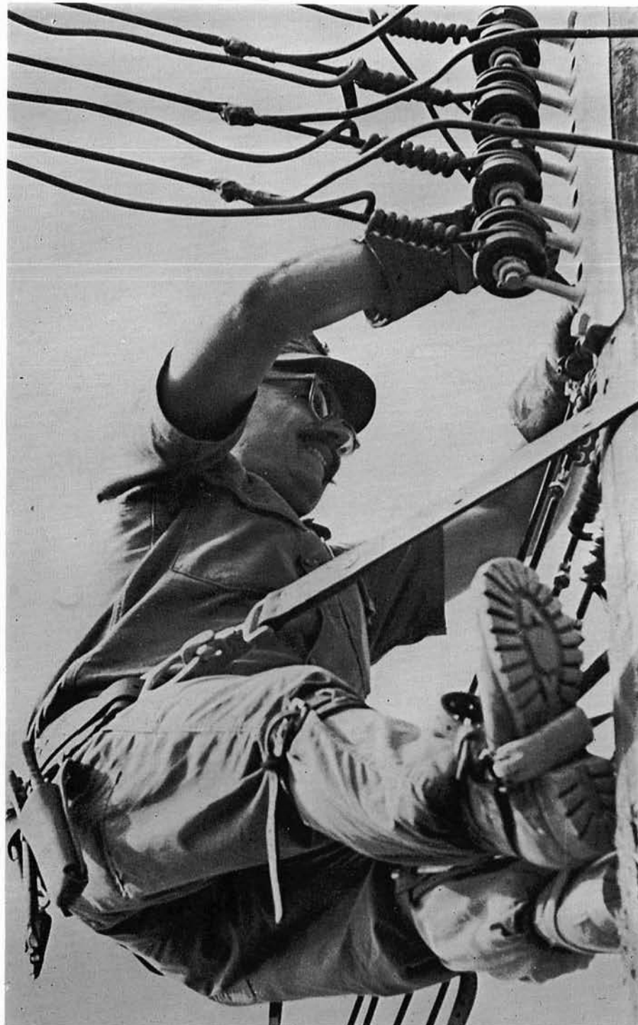
CE1 DEAN helps install power distribution system during our early camp development.
