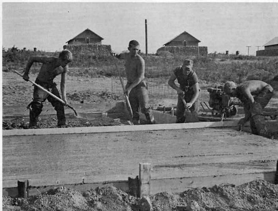
CN SHEARIN, BULCN McCOMBS, SWF2 WOOD and SWF2 BIRDSONG prepare a concrete platform for the CBMU 301 water tank.
