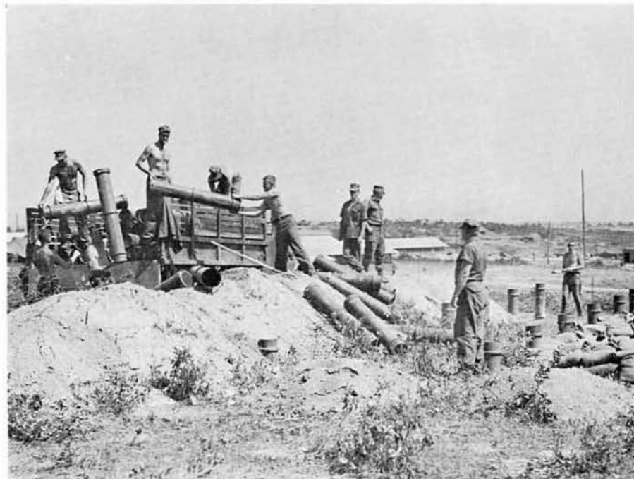
The 175mm gun powder cannisters are used as foundation piers and to cover mortar trenches.
