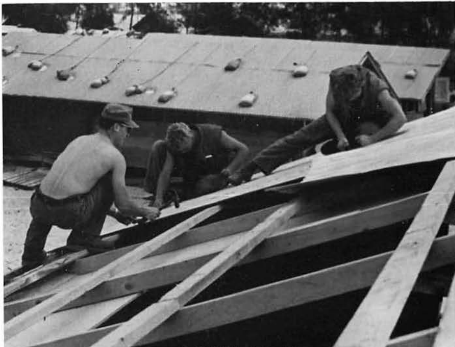
EAS2 FARAONE, BUL3 BIRDSONG and CN KEPNER put tin on the roof of a hut.
