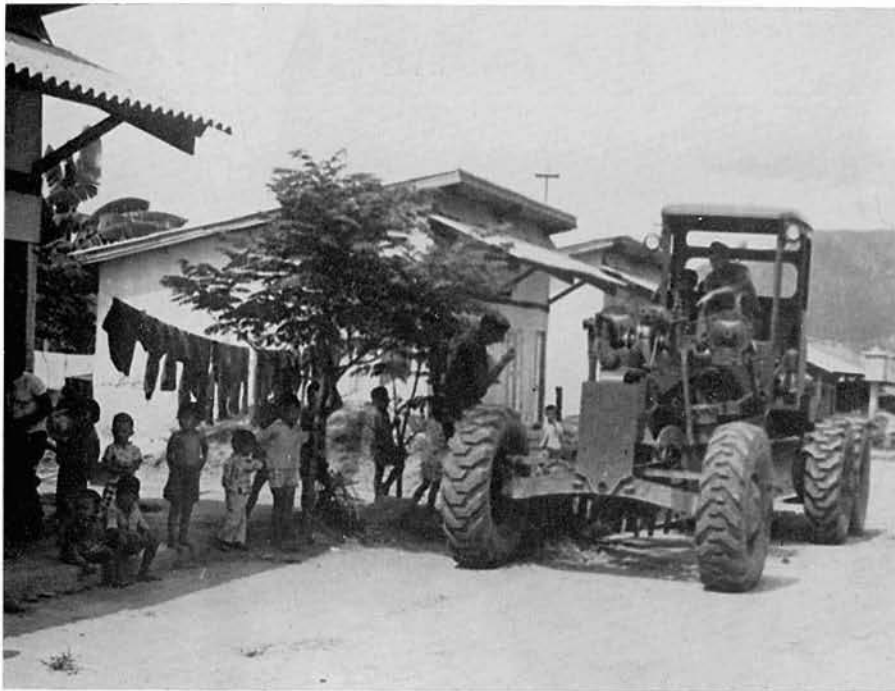
A civic action project near An Hoa provides this village with a new pipeline.
