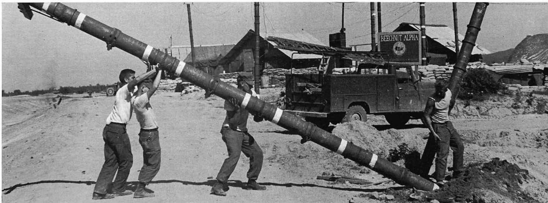
The electrician's CEP2 DIBELKA, CET2 ULMER, CEP2 BEEL and CEW3 OLSON, set a cannister pole.
