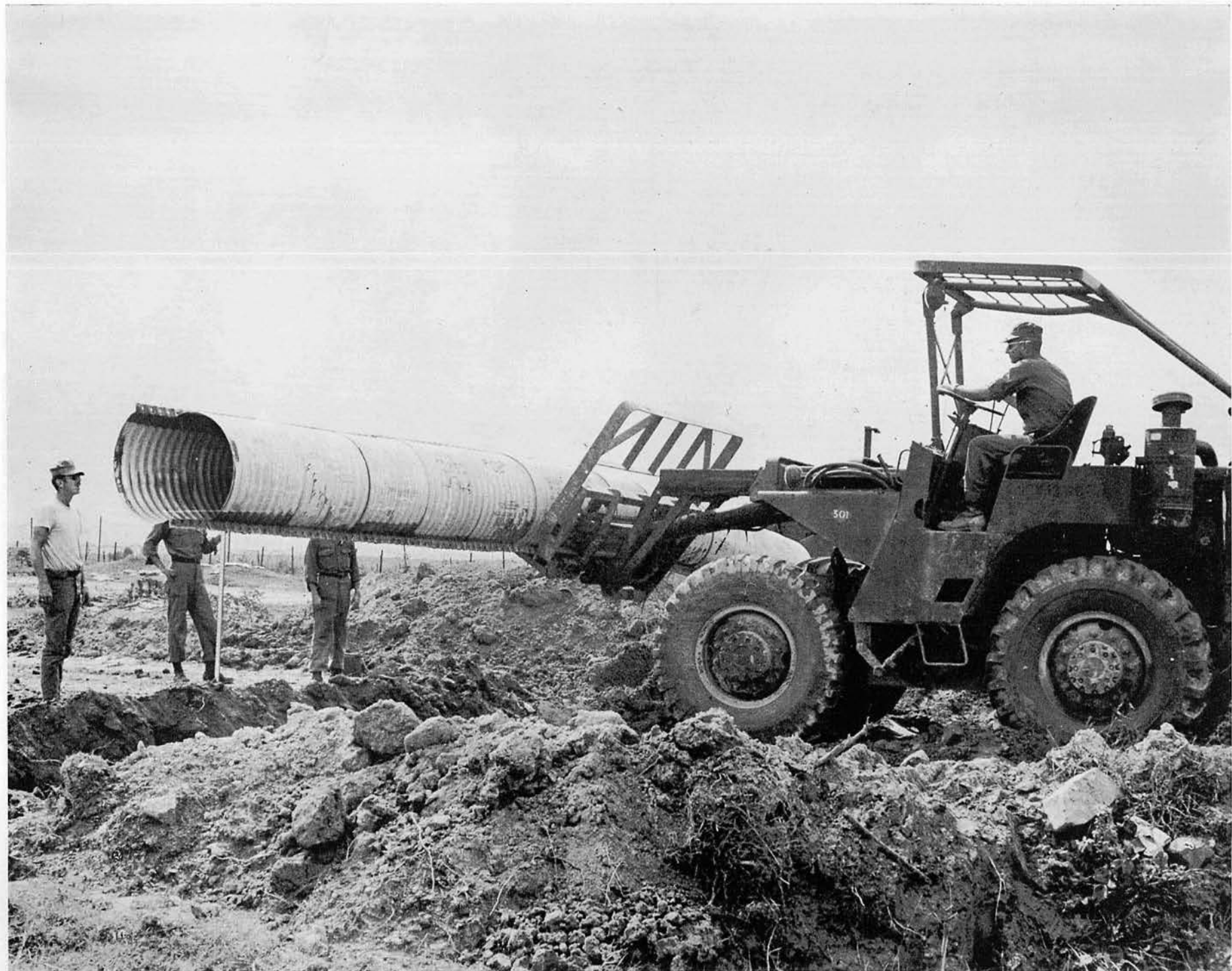
EOC BERTLES lowers a culvert near the French road, west of camp, as EON3 PICARD , EONCH WILLIAMSON and EONCH CRUZ stand by to guide the corrugated pipe.
