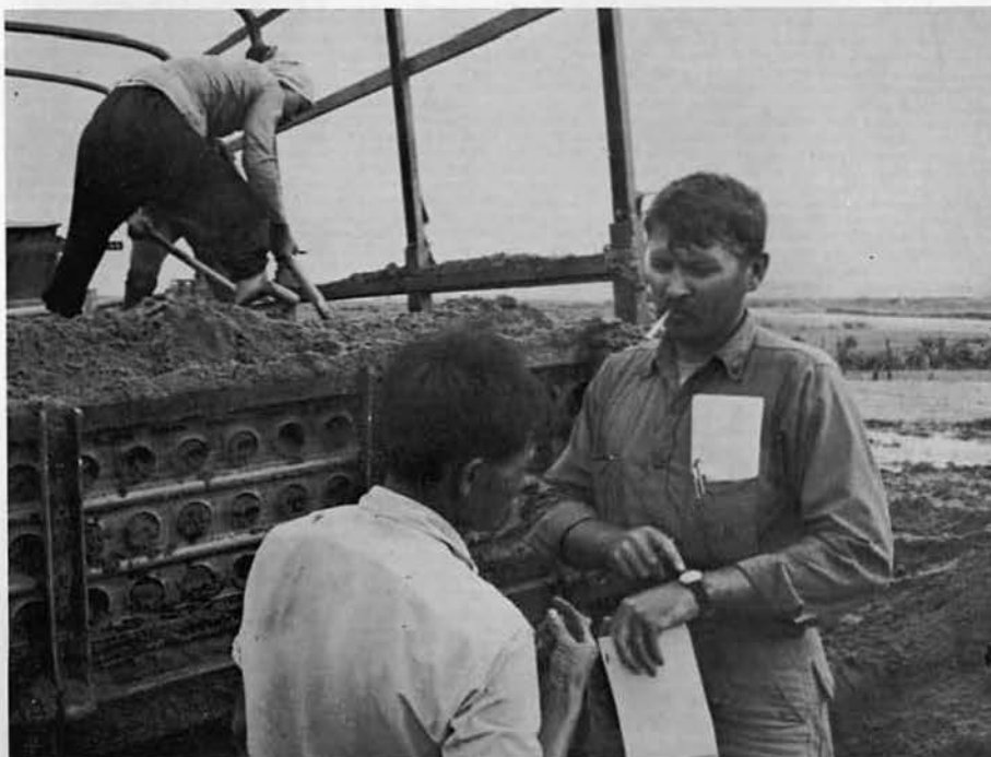
EAD2 SHILLER explains the virtues of a prompt schedule for sand deliveries. It was used for making concrete.
