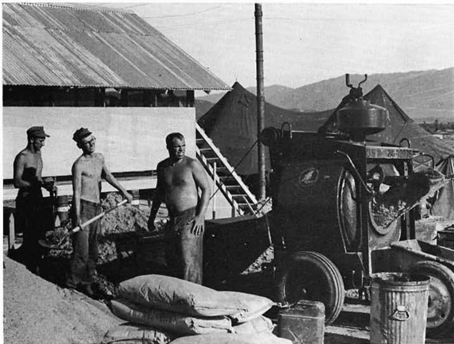
BUHCN TURK, CN PRITCHARD and BUH2 BRAVER mix concrete for a bunker.
