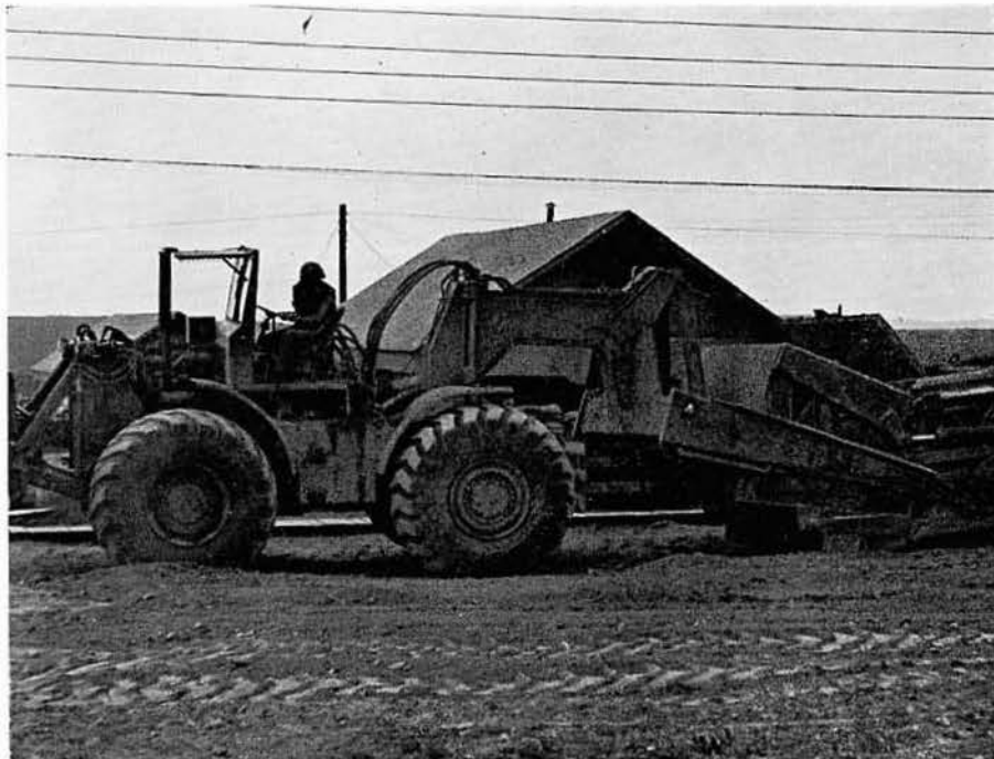
The MRS tractor levels the area over the originally proposed C. P. site.
