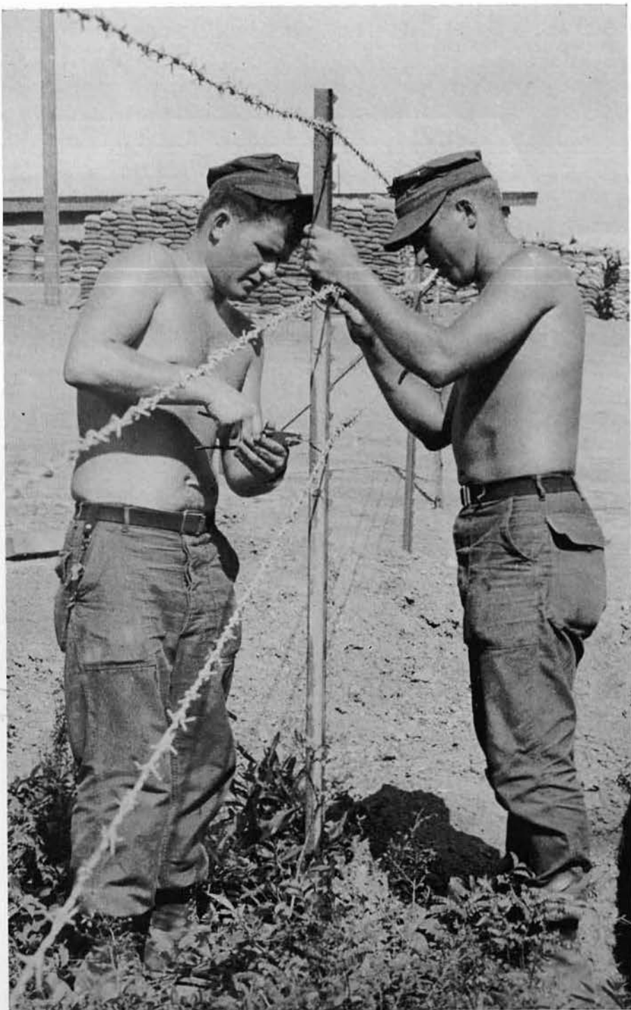
SWE3 SWEAT and SWF3 McMINN constructing boundaries for the outdoor supply yard.
