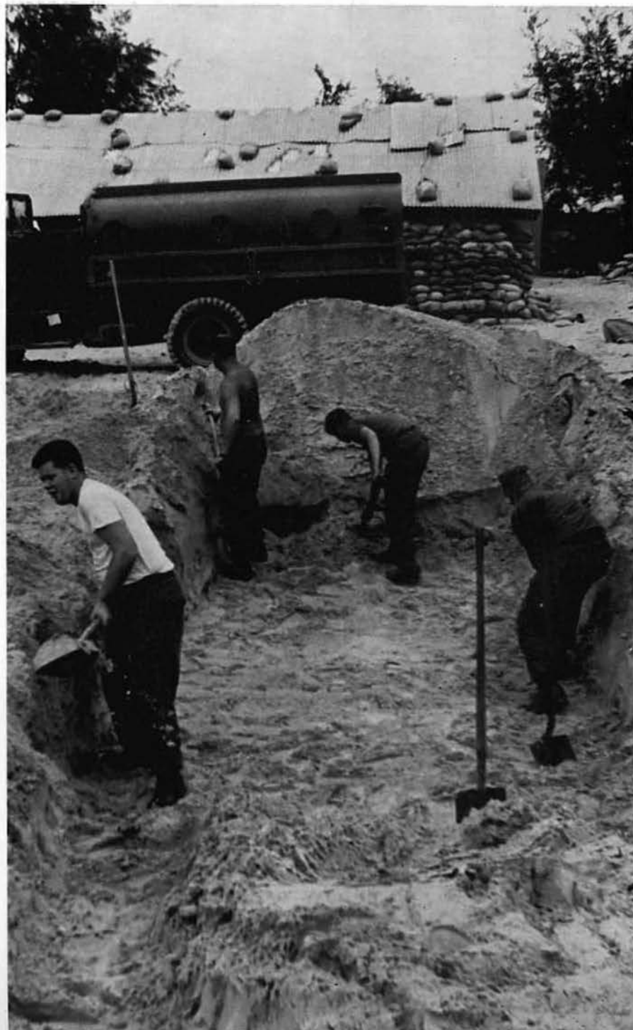
CN HAFFORD, BURCN LLOYD-DAVIES, BUL3 HOPKINS and BUH2 OWSEY dig a hole for a bunker.
