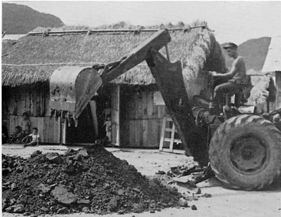
EON2 BROWN works on the water distribution system that will serve domestic functions.
