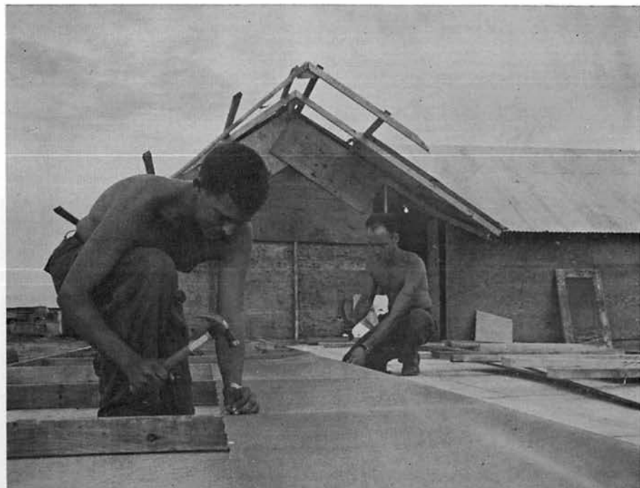
BUL3 KELLY and CEW2 MEEKS prefabricate a wall for the operations office.
