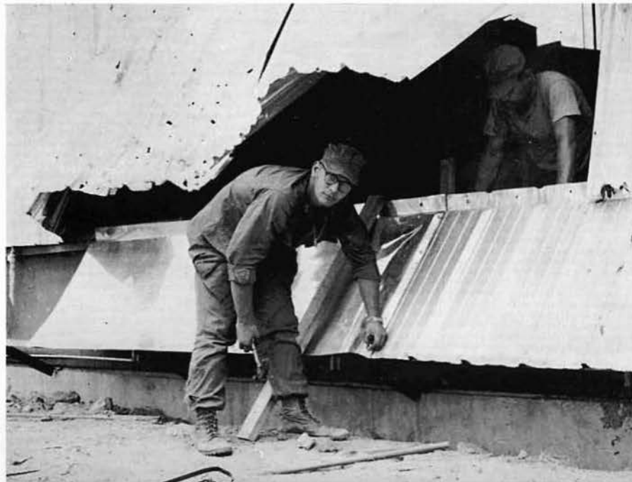
SWE2 BORTMAS helps repair a Marine butler building damaged by rocket concussion and shrapnel.
