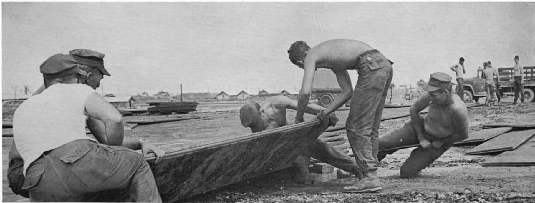
The steelworkers manhandle a stubborn piece of runway matting into place on the Dong-Ha Airstrip.
