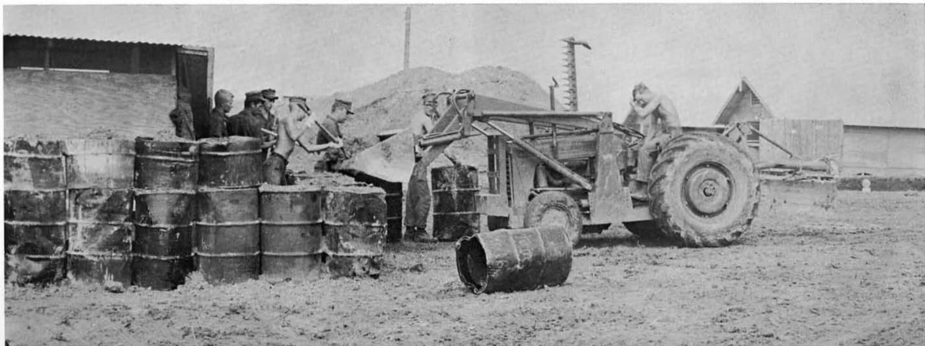
When you run out of sandbags, empty oil barrels filled with earth serve the same purpose.
