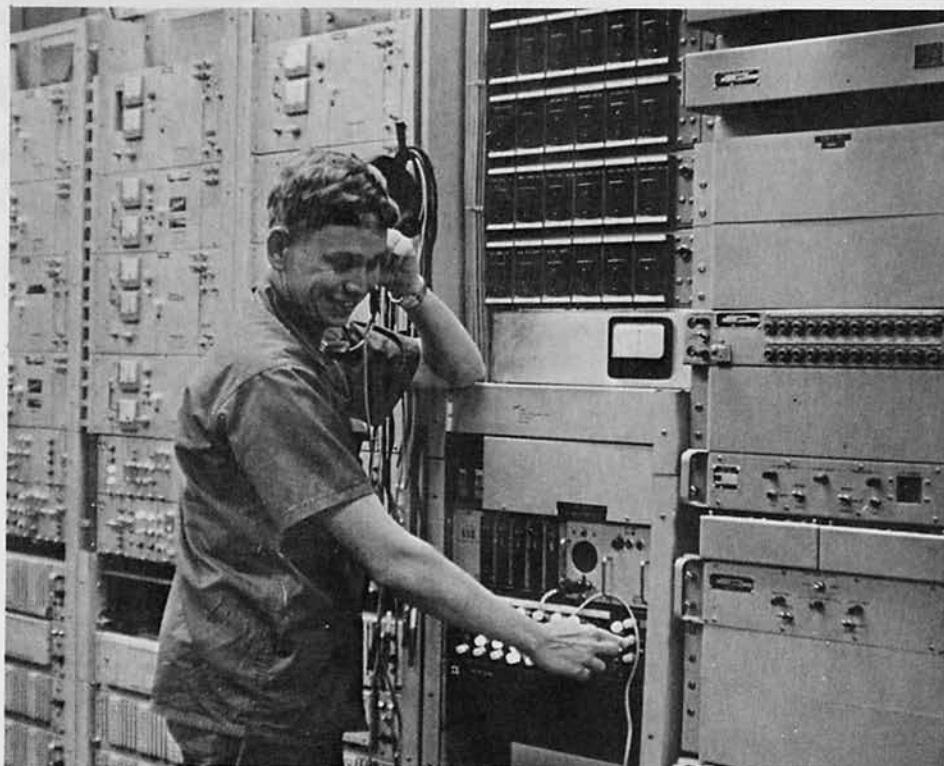
Above, left: RM2 B.R. Hatton of the Triangle Communications Center Control Division troubleshooting a microwave antenna.
