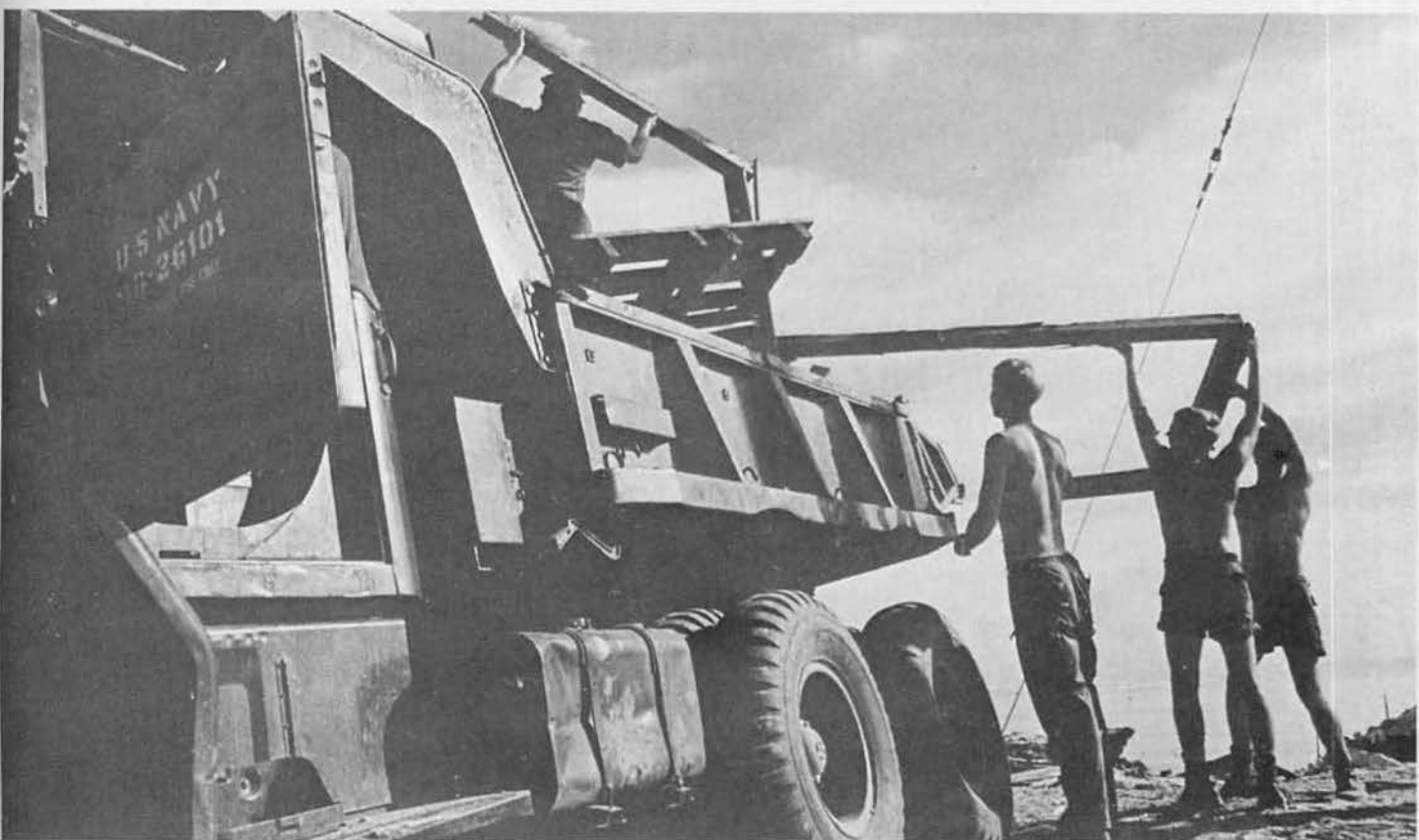
Below: men from "X" Division load scrap lumber and pallets aboard a dump truck for disposal.
