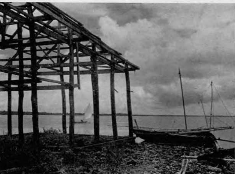
Only the sturdy skeleton remains of this old copra warehouse after the lusty typhoon of 1944.
