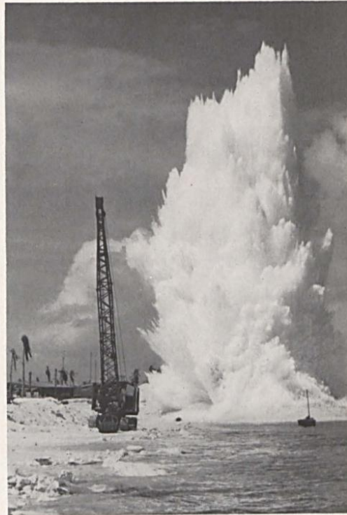
A towering geyser of water rises as a heavy coral shelf is blasted. The blast will give access to the coral sand below the shelf, a valuable material for building good airstrips.
