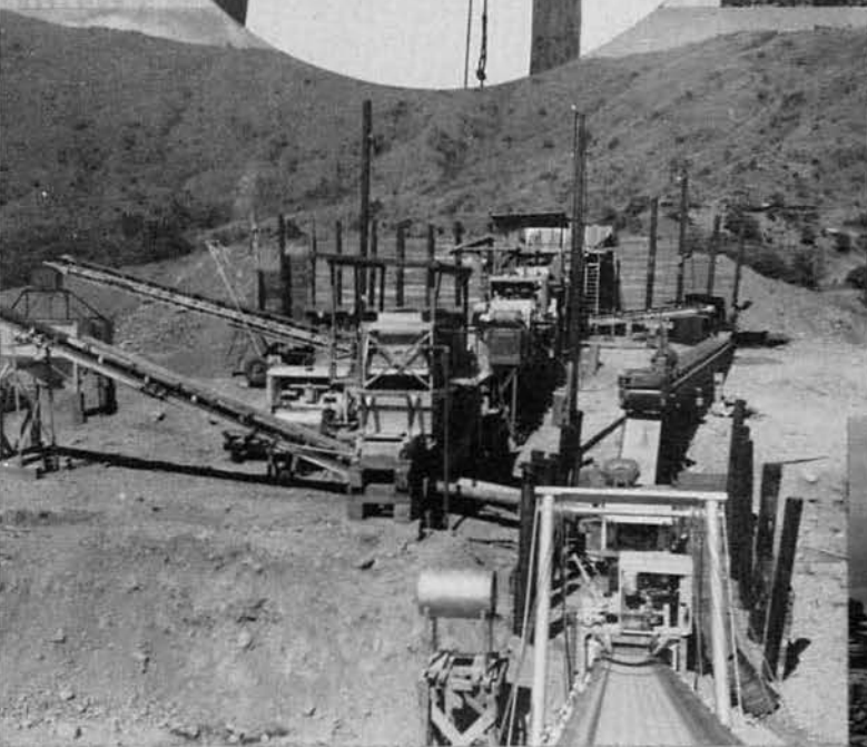
● WEST QUARRY ROCK CRUSHER
