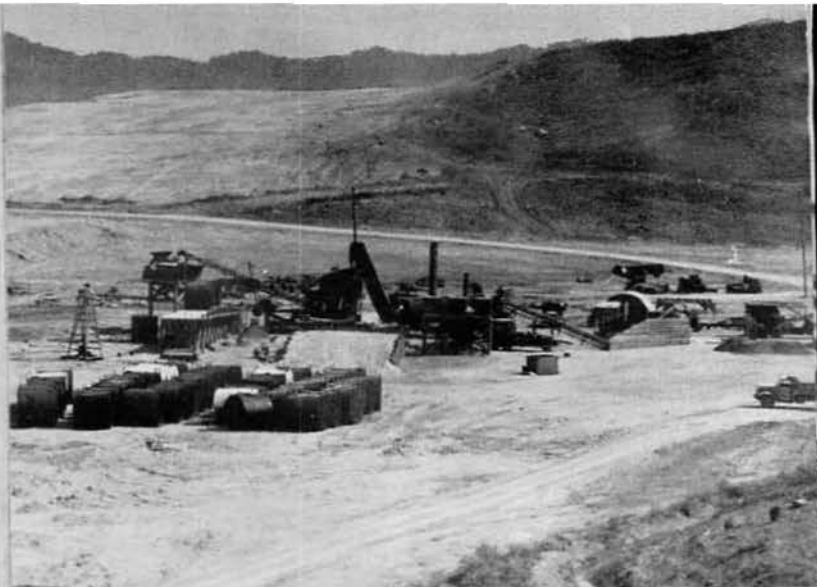
● ASPHALT BATCH PLANT ●
