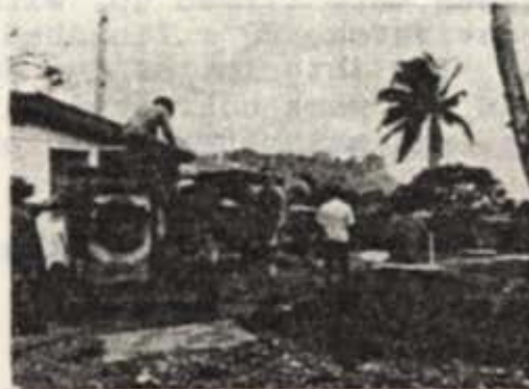
Members of Seabee Team 0420 and local civilians in a concrete crew on Ponape.
