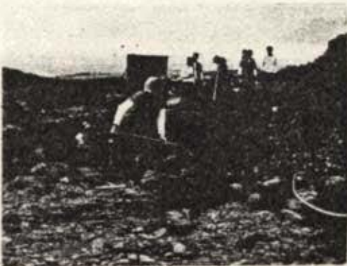
Personnel of NMCB FOUR's Adak Detachment work on the center pad for the T-2 antenna.
