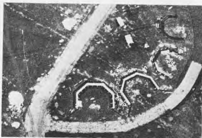
Octagonal revetments under construction. Sides are timber, filled in with coral and earth. Alternative method is to create protective bulwarks by raising earth and rock mounds. Revetments built of cement are not common in Central and South Pacific area
