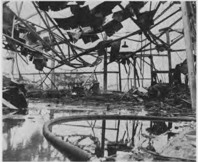
Air blast from explosion at NAS Norfolk shattered this building which stood inside the immediate disruptive area of explosion
