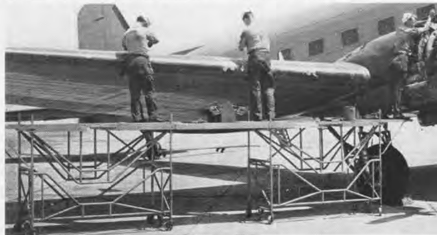
END TO END . WITH CATWALK BETWEEN, WORKMEN CAN SERVICE THE WINGS AND ENGINES OF AN R4D
