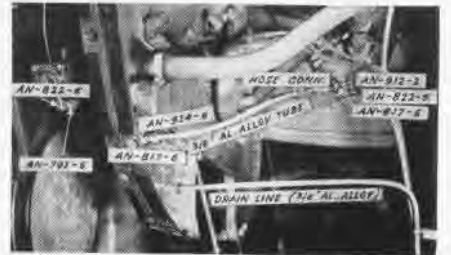
OIL SUMP OUTLET STOPS ICE FORMATION
