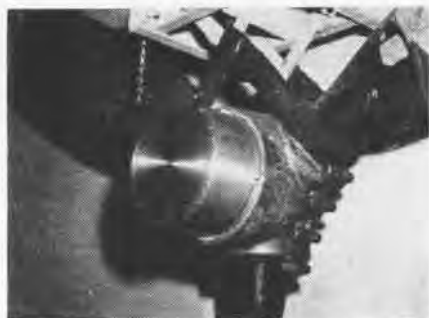
SURVEYED PROP DOME CATCHES OIL DRIP
