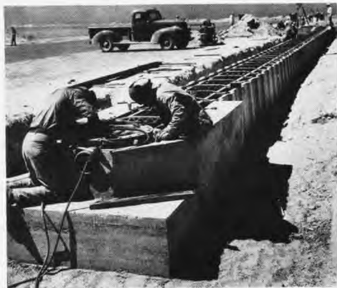
Assembling collecting pot on Hades-Rapex (Mk 3) installation; Fuel from 16 vaporizing tubes feeds into 8-inch burner pipe
