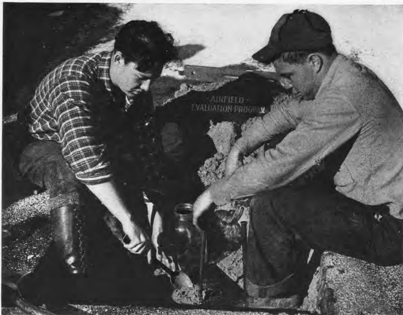
PAVEMENT ONLY AS GOOD AS ITS FOUNDATION LAYERS ALLOW. "GOPHERS" REMOVE SUBBASE SOIL FOR FIELD DENSITY TESTING
