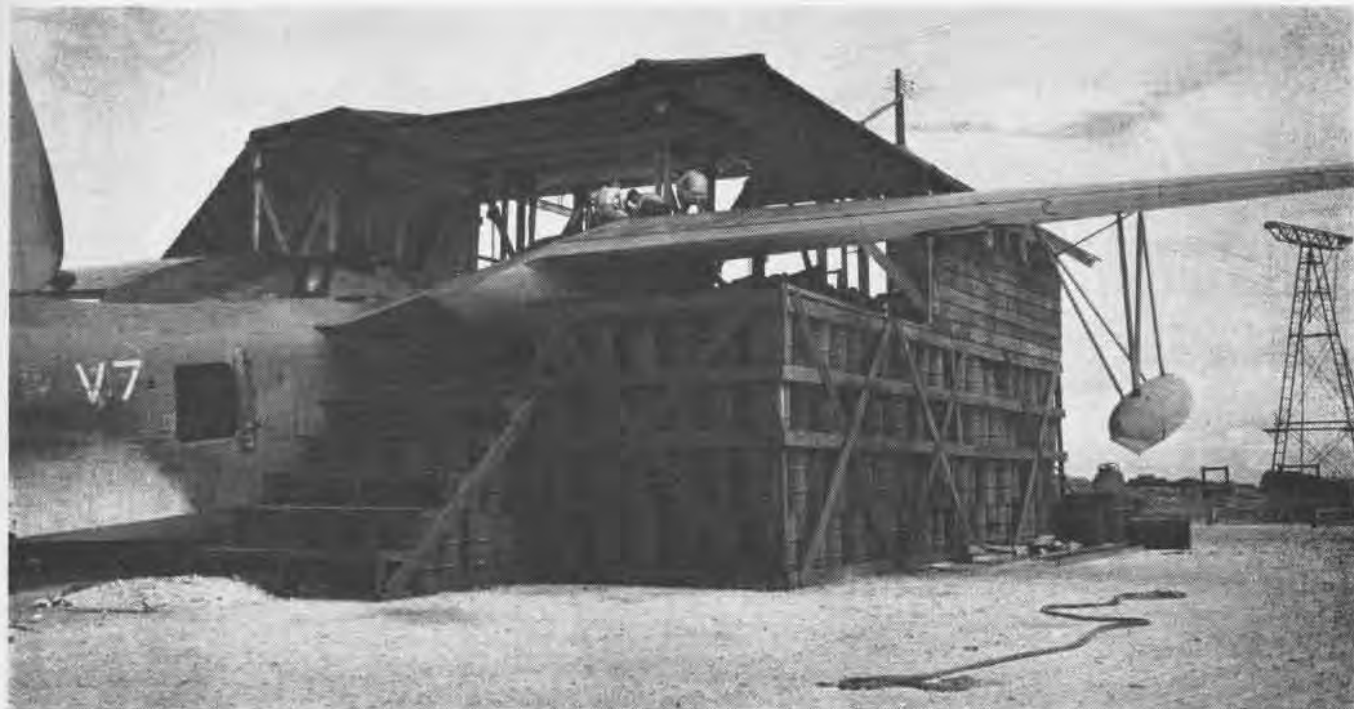
OIL DRUMS HAD TO PINCH-HIT FOR LUMBER IN THIS INGENUOUS NOSE HANGAR FOR P8M MAINTENANCE AT OPERATION CROSSROADS
