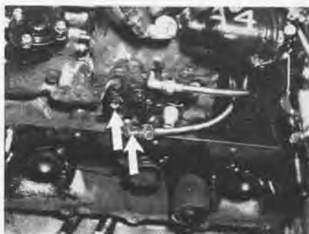
POOR SCREW-IN FAILS TO HOLD ELBOWS
