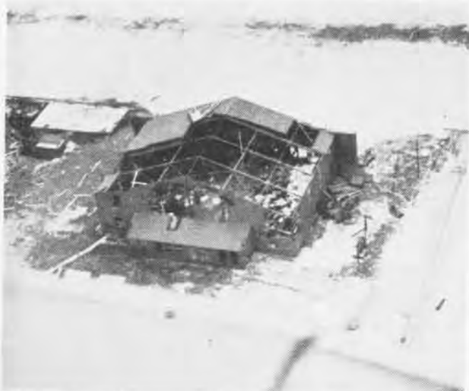
Navy survey plane spotted this devastated hangar at Boca Raton air field; Storm damaged many buildings, no lives lost
