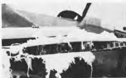
BLAST DAMAGE LEAD TO THIS BAD CONDITION
