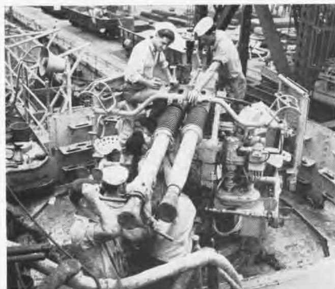
Activation team reinstalls gun barrels on a 40 mm. mount preparatory to placing mount in service again on the Cabot
