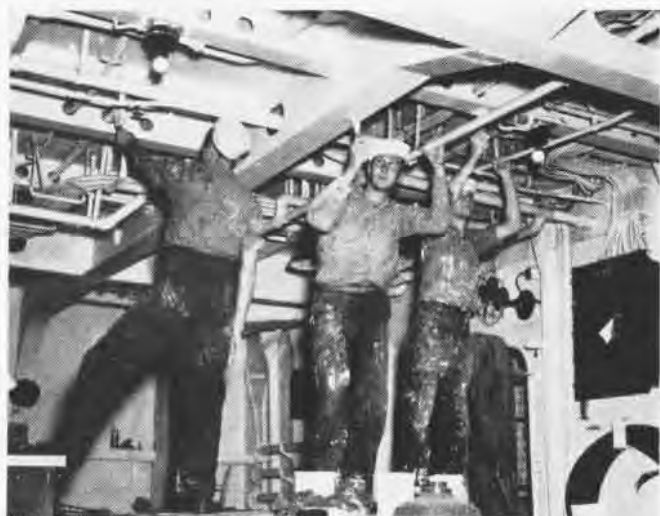
Activation crew below decks on Cabot paint the overhead in the chief petty officers' mess preparatory to opening it up
