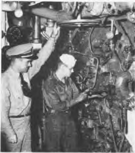
R. J. Murray, ADC, and J. W. McCrory of Cabot's crew light steam boiler
