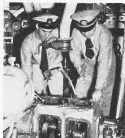
B. Restuccia, MMC, and R. J. Murray examine high pressure air compressor
