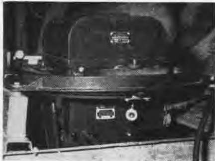
A CLOSEUP OF THE INSTALLATION USED IN R5C
