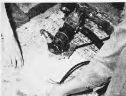
FUEL TRANSFER PUMP USED IN DEFUELING JOB
