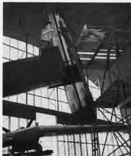
In hangar at North Island K. F. Abbott, AM2, makes repair on rudder of PBM of VF-731
