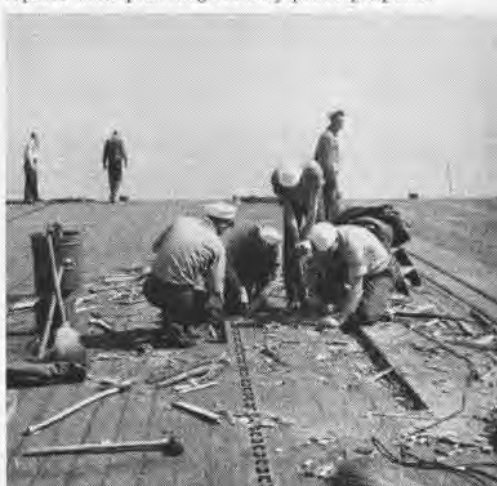
DECK REPAIRS aboard Bon Homme Richard replace deck planking torn by plane propeller
