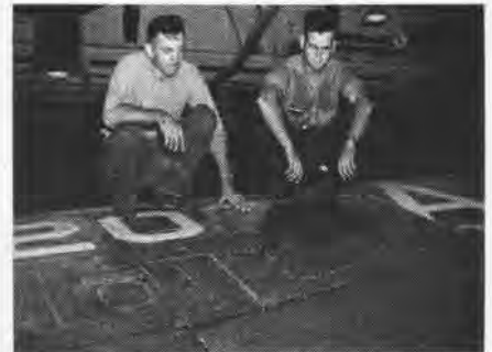
ONCE TERMED non-repairable, a hole in the wing of a Corsair fighter measuring 44"x43" was repaired by Minnard Rudd and Clarence Russell, both AM1's, with the Boxer's all-Reserve air group off Korea. The plane was in flying condition 1.2 hours later.
