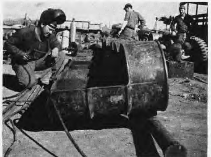
SEABEE Rodgers developed gravity flow avgas supply ramp at the airstrip, using empty gas drums, to fill gas truck in 8 minutes
