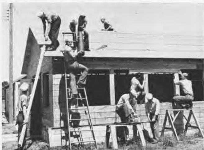
CARPENTERS, too! Holmes, Empey, Hatzenbubler, Weitstein, Alexander and Holman work on combined shop and storage building
