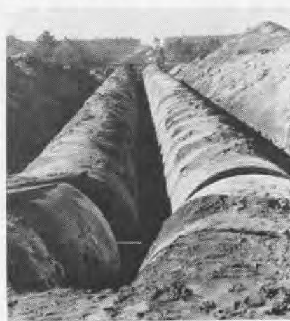
66" CONCRETE DRAINAGE PIPES AT SAUFLEY
