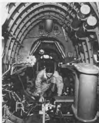
DURING the flight, Paul Munchus monitors the equipment installed in aft section of the P2V.
