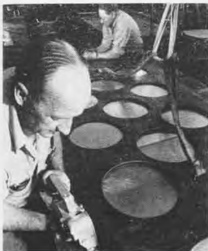
WITH a metal pattern clamped into place, electric shears cut the sheet to the required size.
