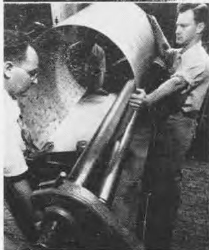
THE PROPER diameter for the afterburner is obtained by passing sheet metal through roller.
