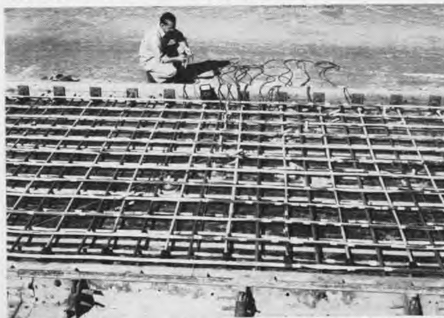
Gauges will measure stress of test weights after concrete has been poured
