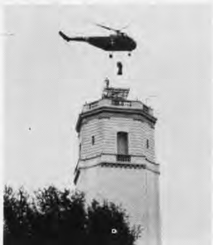
WHEN NO CRANE was available to hoist a 1250-lb. pedestal for "Storm Detector" radar to top of 125 ft. tower at Barksdale AFB, an Army 'copter from Ft. Hood, Tex. took care of it.
