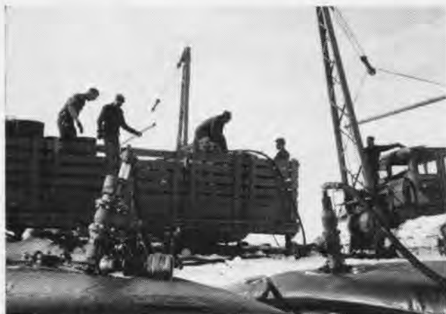
DIESEL FUEL IS PIPED INTO 800-GALLON, SLED-MOUNTED TANKS
