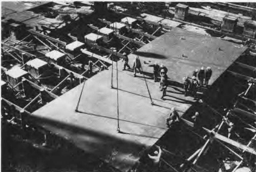
WORKMEN LAY the first keel section of the world's first nuclear-powered aircraft carrier, the Enterprise (CVAN-65), at the Newport News Shipbuilding and Dry Dock Company. According to the Secretary of the Navy, the Honorable Thomas S. Gates, Jr., the name perpetuates the WW II carrier and her six predecessors. The new ship's eight reactors will give her a normal steaming period of more than two years before replenishment of her nuclear fuel.
