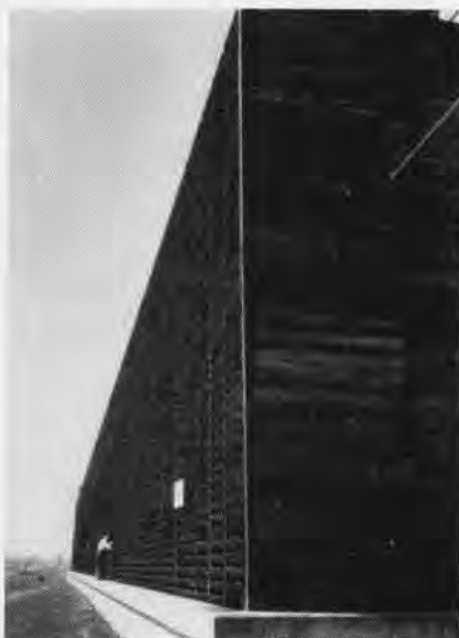
EXHAUST-HEATED WATER IS COOLED HERE
