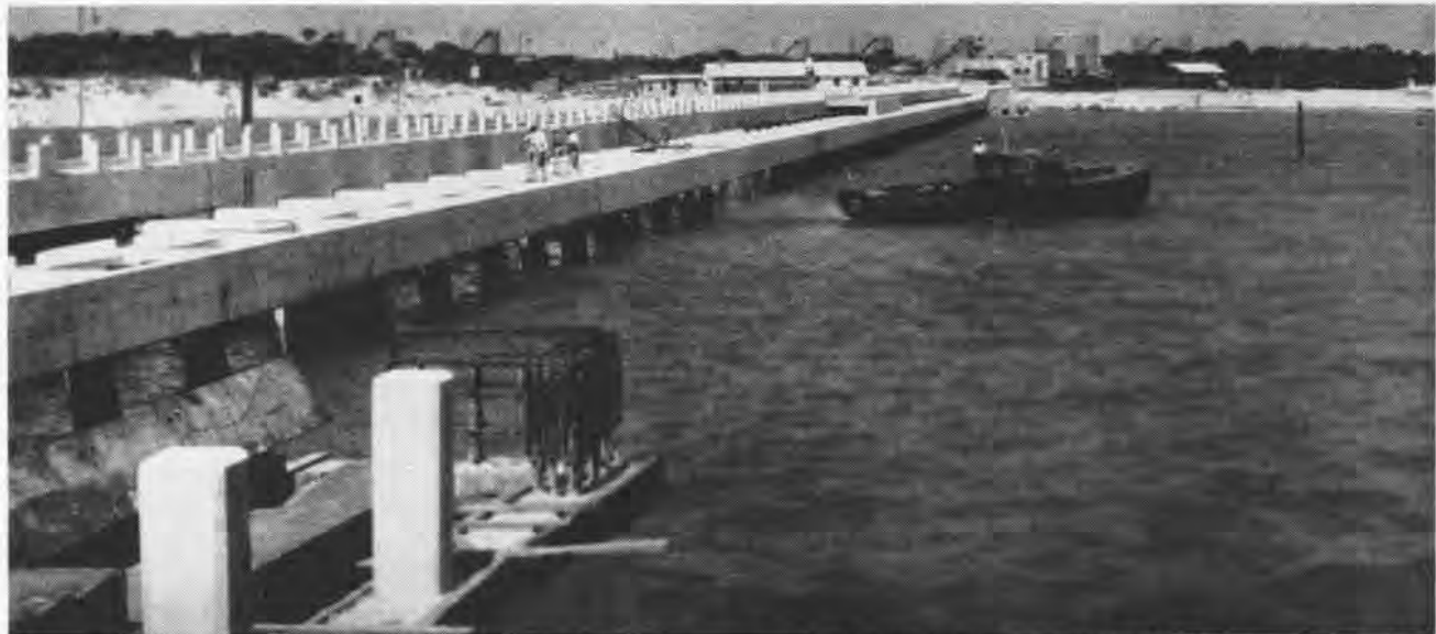
THIS IS THE SEAWARD END OF THE PARTIALLY COMPLETED FUEL PIER AT THE SITE OF THE FUTURE NAVAL AIR STATION AT ROTA
