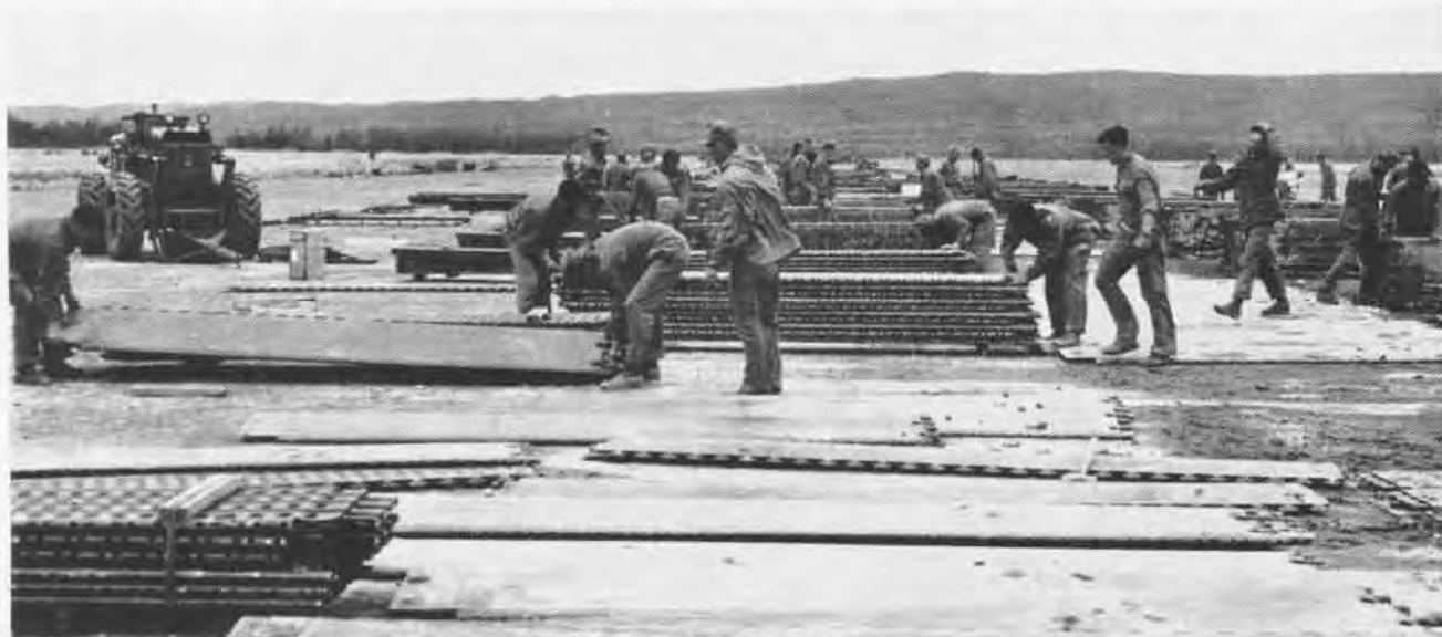
STRIP, 3400 FEET LONG, 60 FT. WIDE, IS BUILT OF ALUMINUM PLANKS, EACH 2 FT. WIDE, 12 FT. LONG, AND WEIGHING 161 POUNDS
