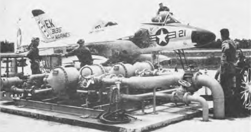
THIS SUPER GAS STATION at Cherry Point is one of several recently completed to expedite refueling operations. Each pump has four hoses and a pumping capability of over 400 gallons a minute. The jet refueling system can handle 32 aircraft simultaneously and launch them in 25 minutes. With the new installation, Cherry Point expects to slice in half the number of man-hours necessary to refuel and to minimize the need for refueler trucks on the Air Station.
