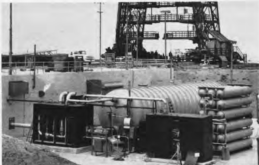
PLS INCLUDES LOX TANK, GASEOUS OXYGEN BOTTLES, PIPES, VALVES HOUSED IN BOXES
