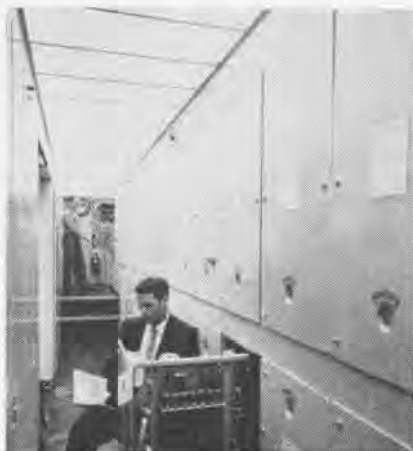
COMPUTER RACKS , the backbone of the trainer, are periodically checked by inspectors.
