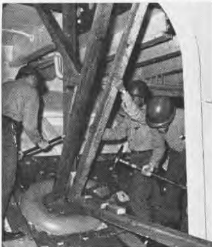
FAILURE of weakened structure is avoided as manhole is shored up against an angry sea.
