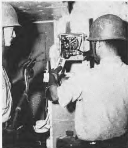
ELECTRICIAN makes sure no other source of power is in use before making the connection.
