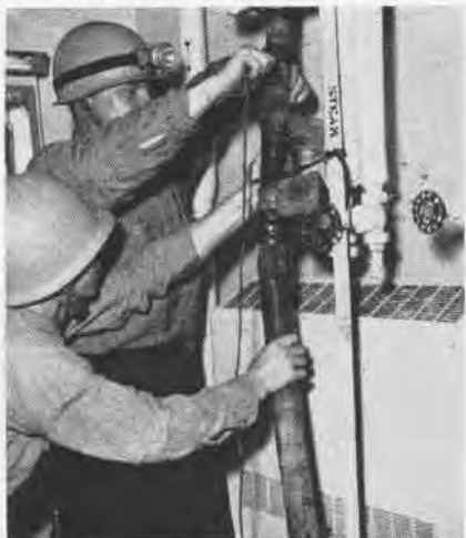
SPEED in applying patch to ruptured water lines prevents flooding and continues use.
