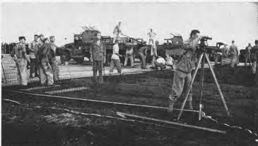
MARINES EXPEDITE building of a runway of matting to set up expeditionary airfield. Short Airfield for Tactical Support (called SATS) can support attack aircraft in limited runway areas.
