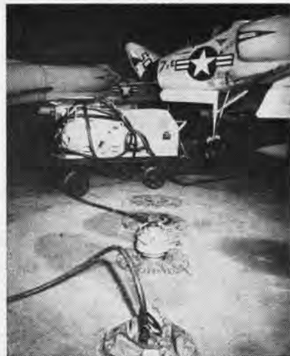
THIS HANGAR DECK HOUSES POWER OUTLETS
